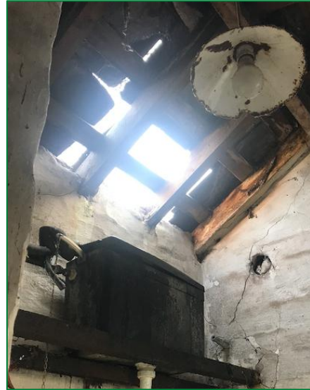
Holes in the roof in the southeast section of the outbuilding
