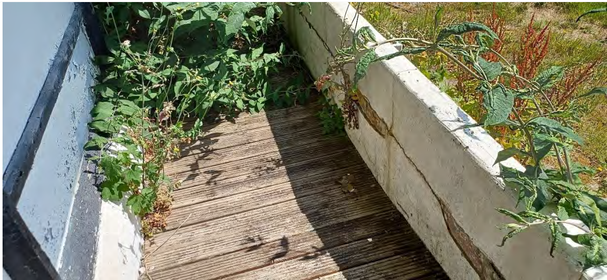
Figure 52 – Hole in boarding, left side, front wall
