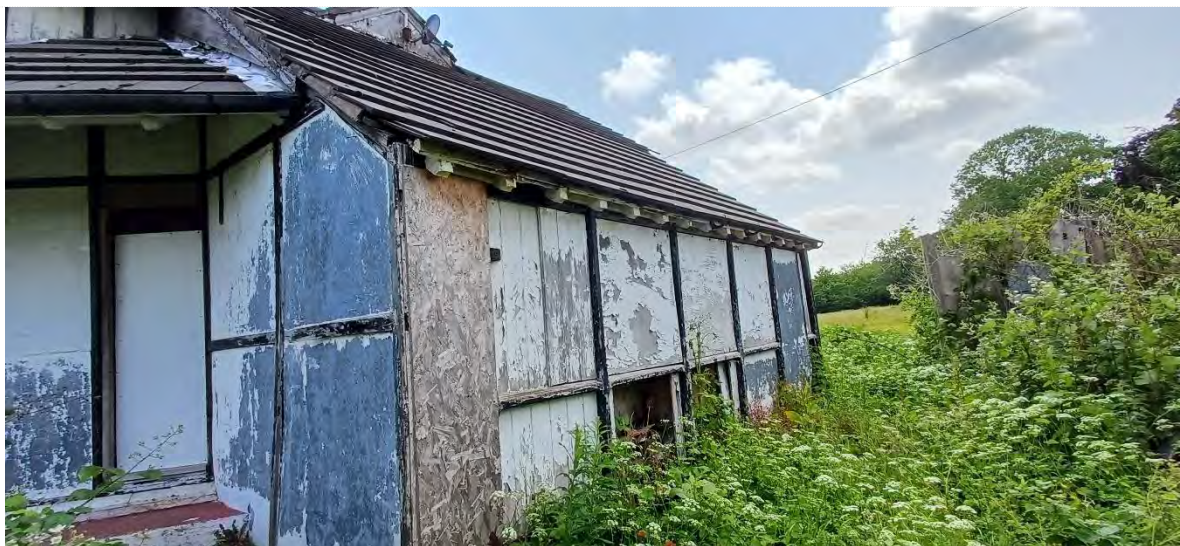
Figure 43 – Missing guttering, rear left corner
