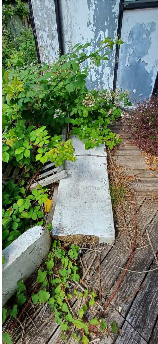
Figure 51 – Collapsed retaining wall front left
