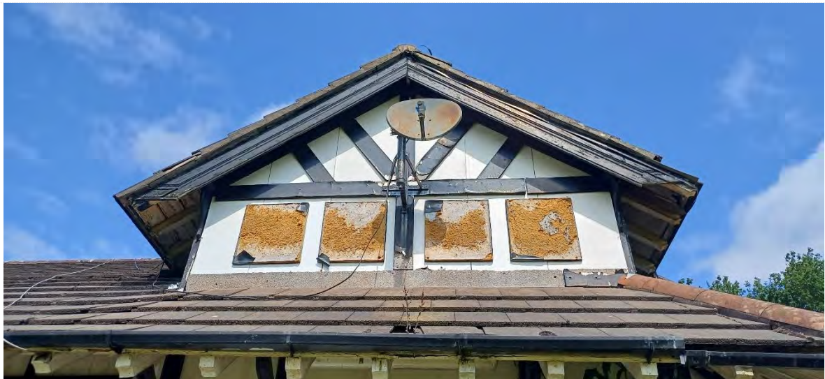
Figure 15 – Misaligned guttering, right side
