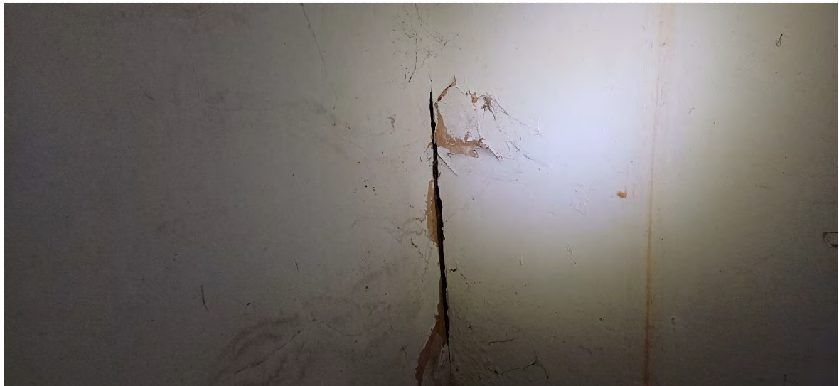
Figure 72 – Rust to beading, rear right wall
