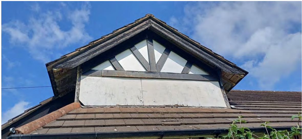
Figure 9 – Gap to render/tiling, misaligned guttering
