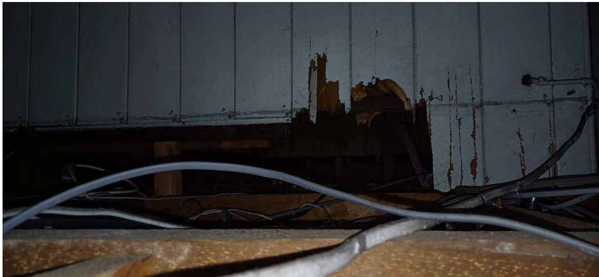
Figure 94 – Damage to ceiling, rear of bar
