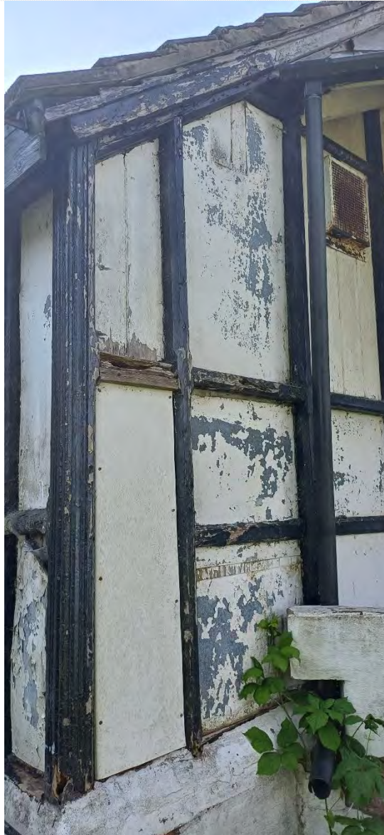
Figure 27 – Rotten timber, right side, rear
