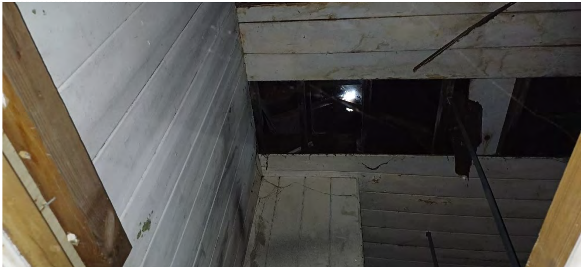
Figure 96 – Collapsed floor, left toilets
