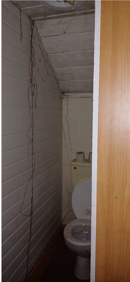
Figure 83 – Vegetation penetrating front left corner
