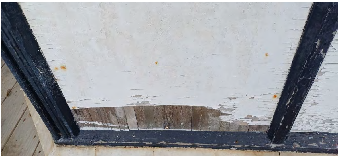
Figure 36 – Rotting timber to centre
