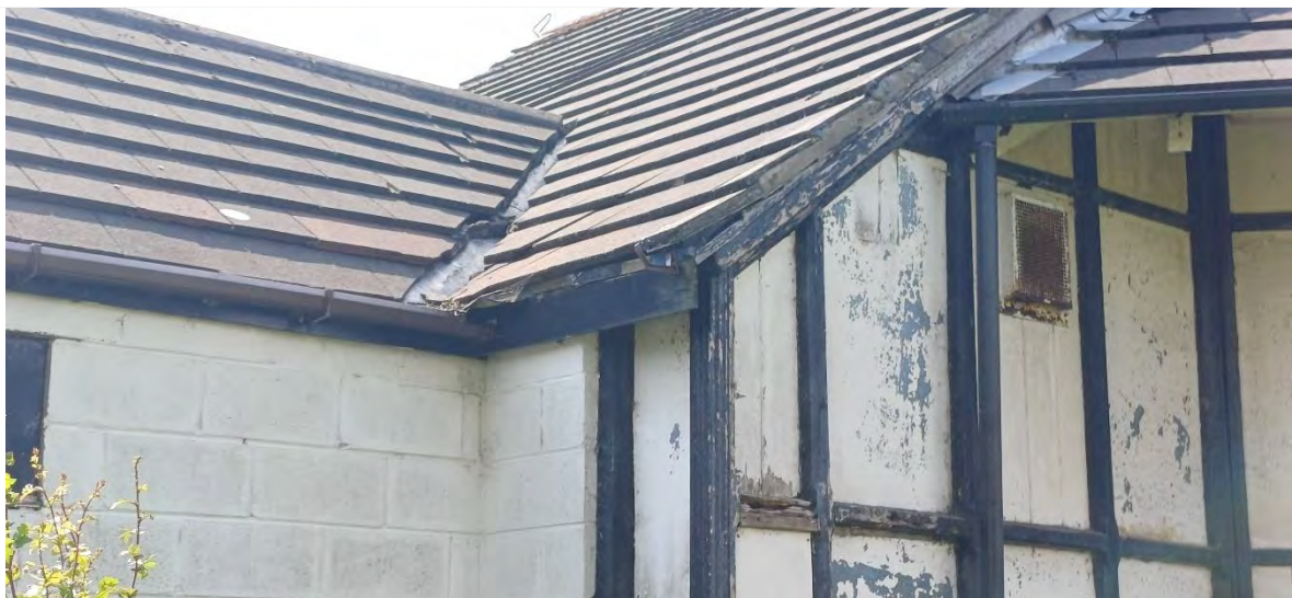
Figure 23 – Missing guttering, right side, rear
