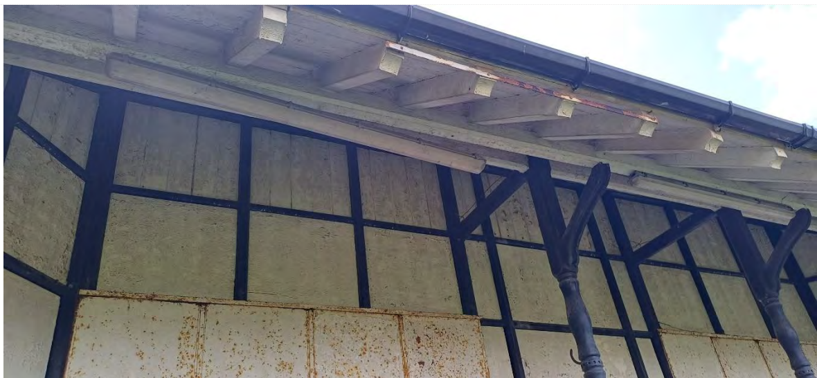
Figure 32 – Boarding to roof, left side of rear right dormer
