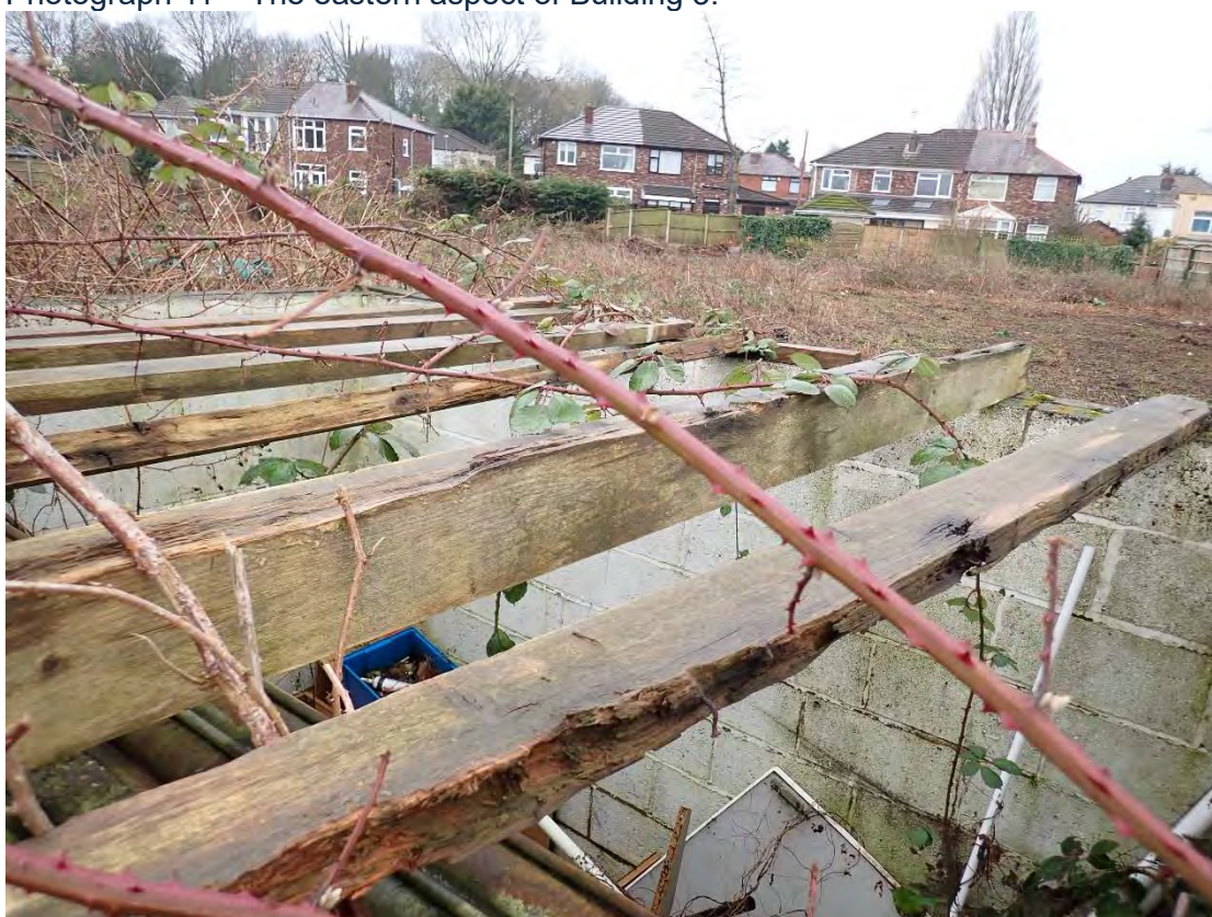
Photograph 12 - Remaining timber rafters on Building 3, showing the absence of a roof.
