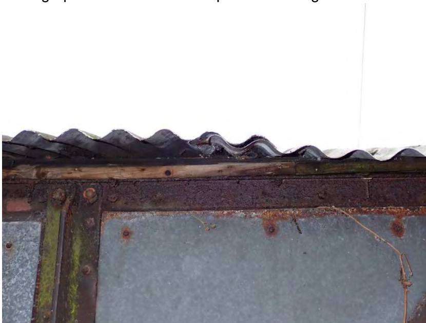
Photograph 10 – A gap between the timber cladding and corrugated roof on Building 2.
