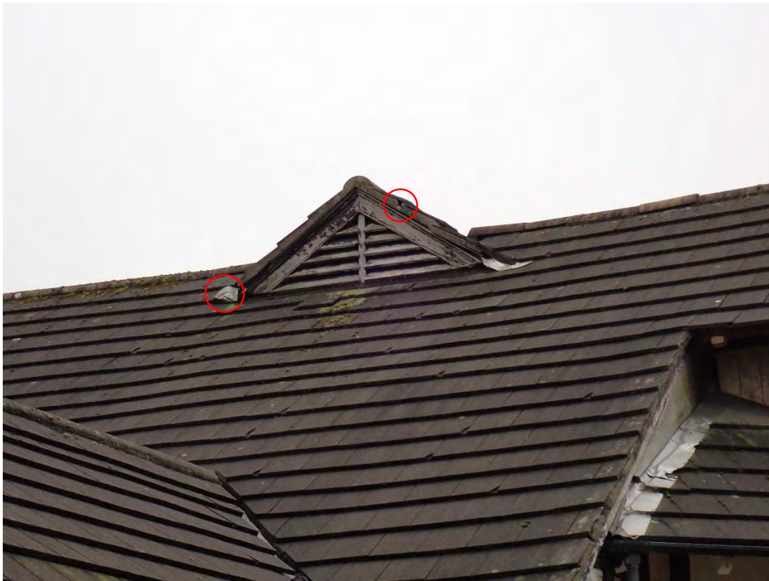
Photograph 5 – Gaps in the mortar of the end tiles and underneath the raised lead flashing on Building 1.
