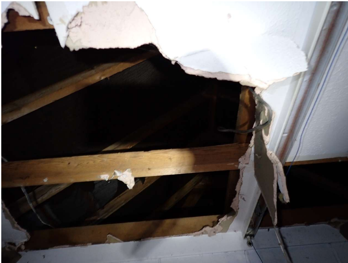
Photograph 17 – Damaged ceiling within Building 1.
