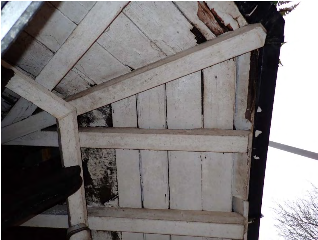
Photograph 7 – Gaps between the bitumen felt and timber which creates a suitable crevice for bats.
