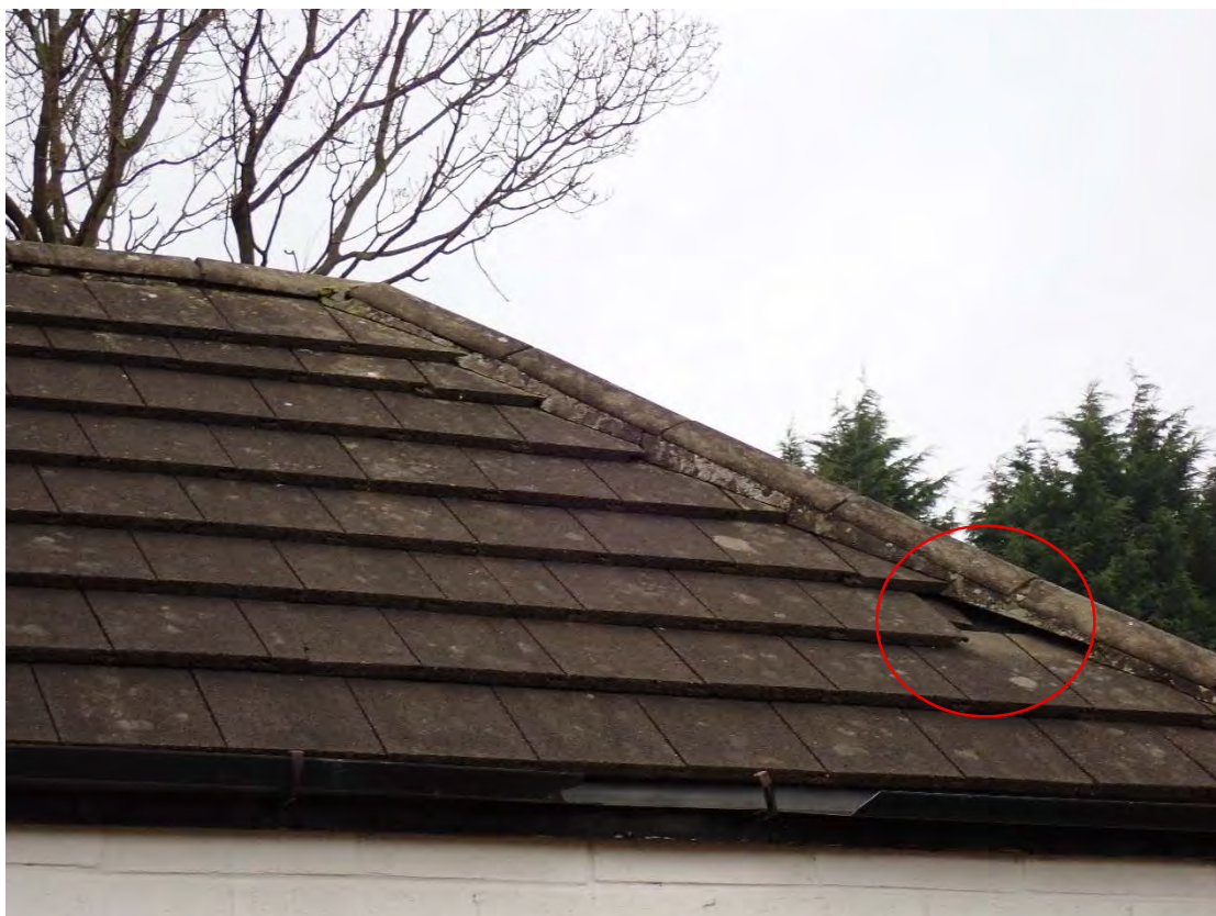
Photograph 4 – Missing roof tile on Building 1.
