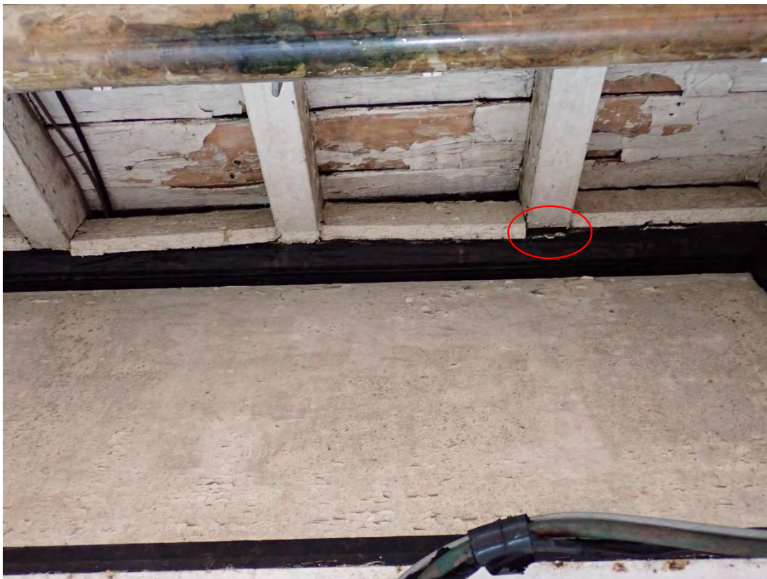
Photograph 6 – A gap in the overhanging porch where the timber connects to the wall plate.
