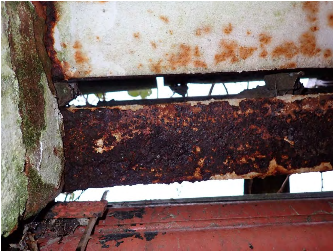
Photograph 13 – Gap above the roller-shutter door on Building 3.
