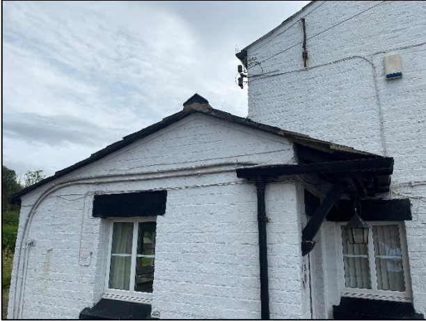
Northern elevation highlighting missing mortar Between roof slates and wall tops.
