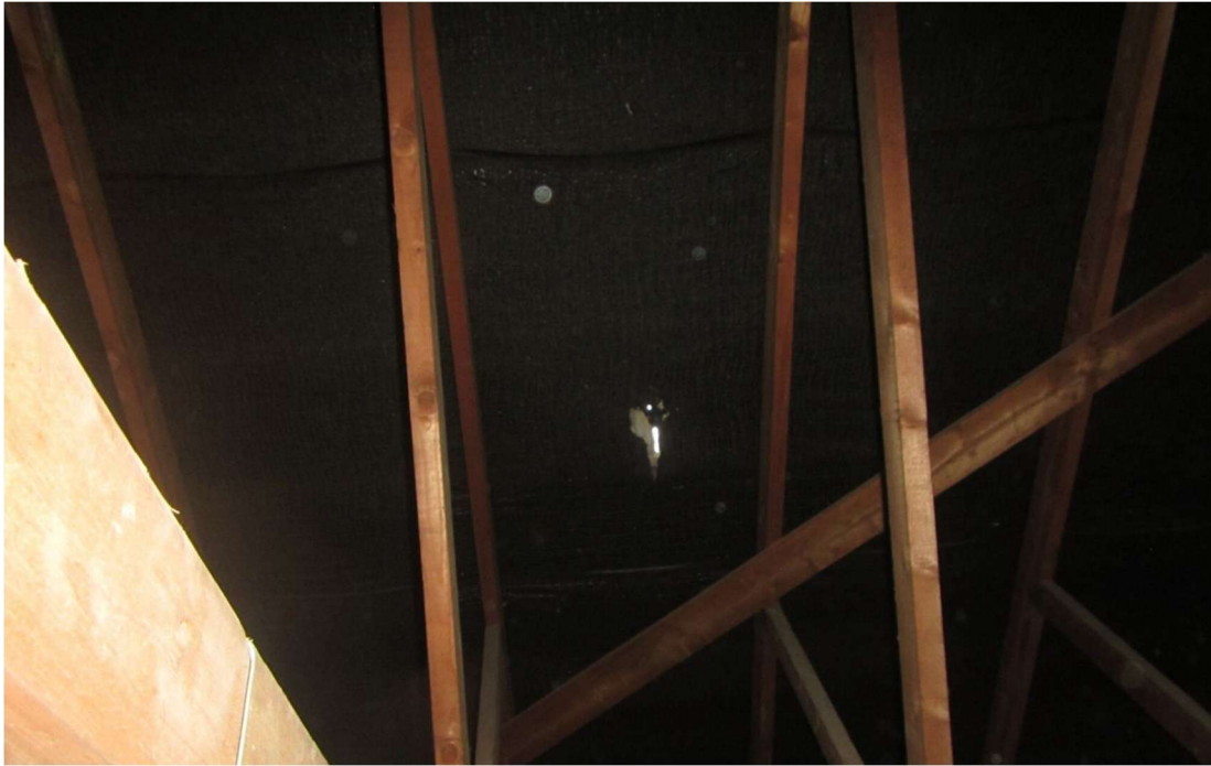
Photograph 23 – Damaged bitumen felt lining the roof of Building 7.
