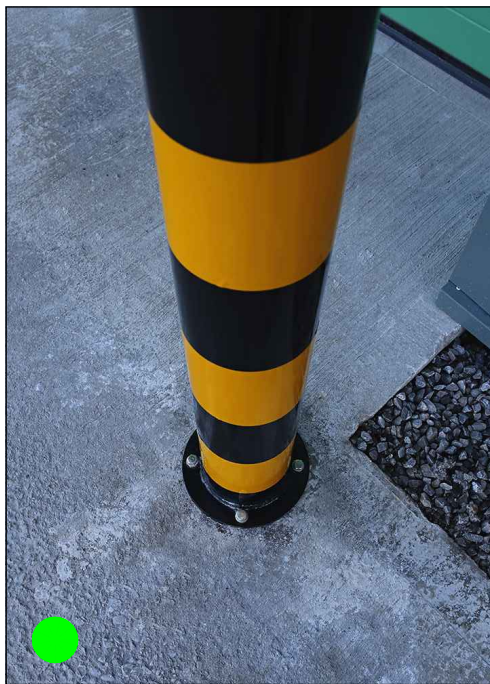
Bollard Type 2 - Impact Protection Steel posts, 1100mm high. Concrete filled, marker painted. Bolted to concrete hardstand.
