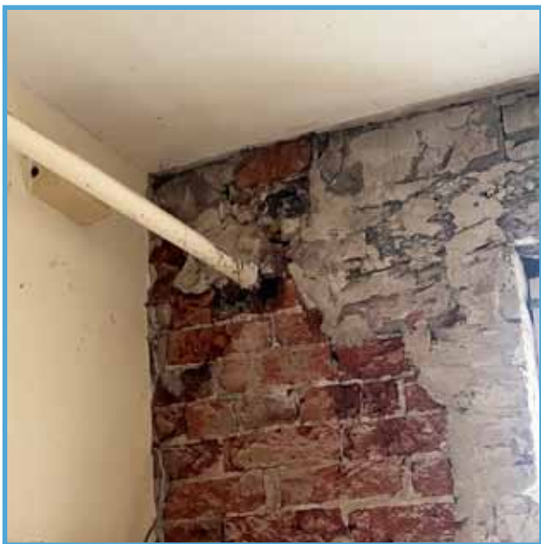
Examples of areas that require new plasterwork
