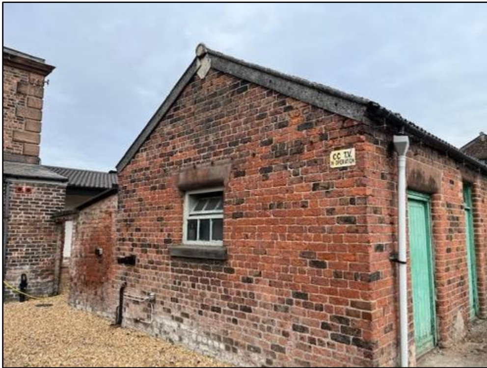
Fig 8: View of the southern gable. The gable is in fair condition, but an obvious entry point is seen at the apex.
