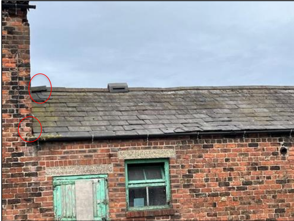
Fig 6: A closer view of the slate roof section. Several displaced tiles have been circled.
