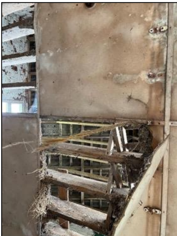
Fig 10: The upper floor of the two-storey section could not be accessed due to obvious rotting and damage. The roof space could be clearly seen despite this. Wooden purlins and rafters support the corrugated asbestos roof.
