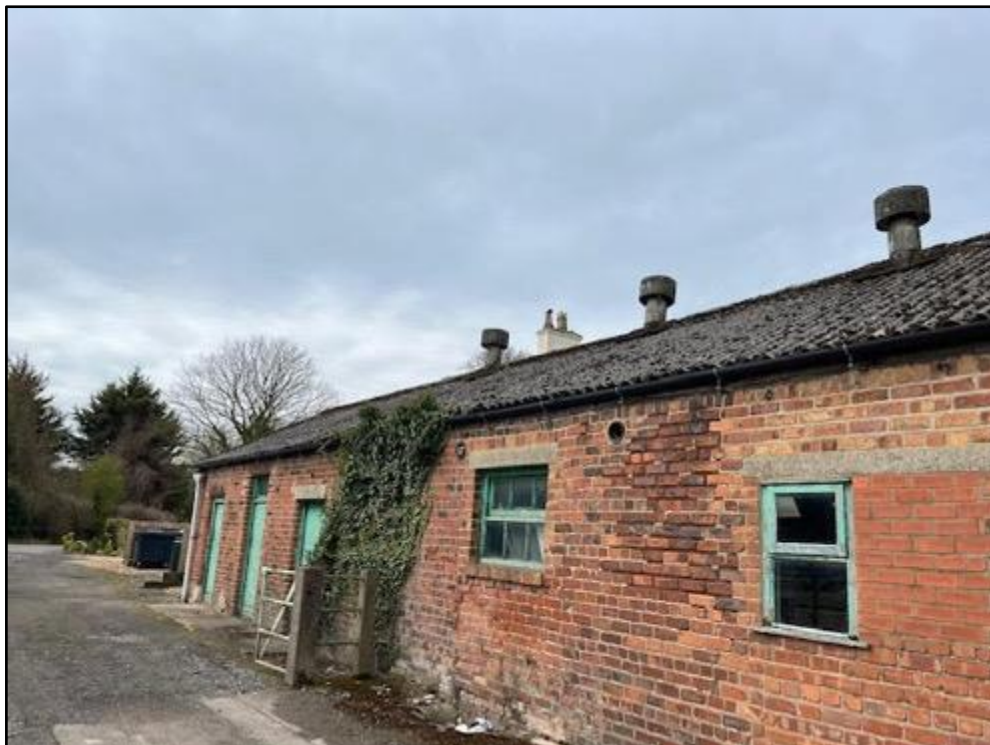
Fig 7: A view of the single-storey section with a corrugated asbestos roof. Windows throughout the building are open, creating ideal access points for foraging bats.
