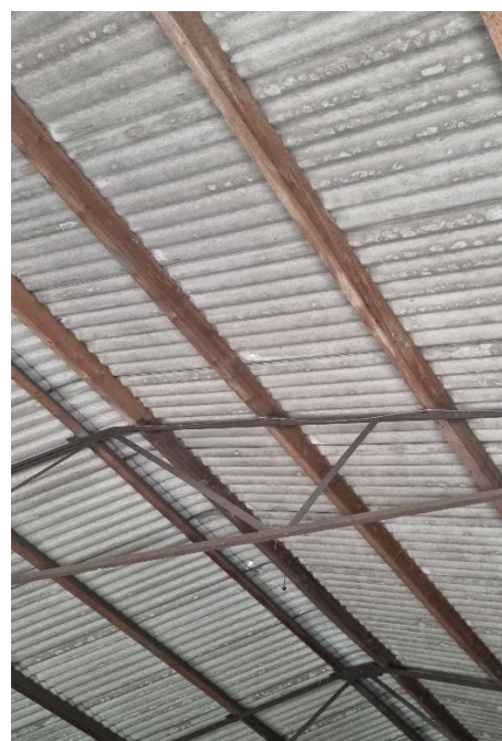
(Holes in the roof – Rusty stanchions)
