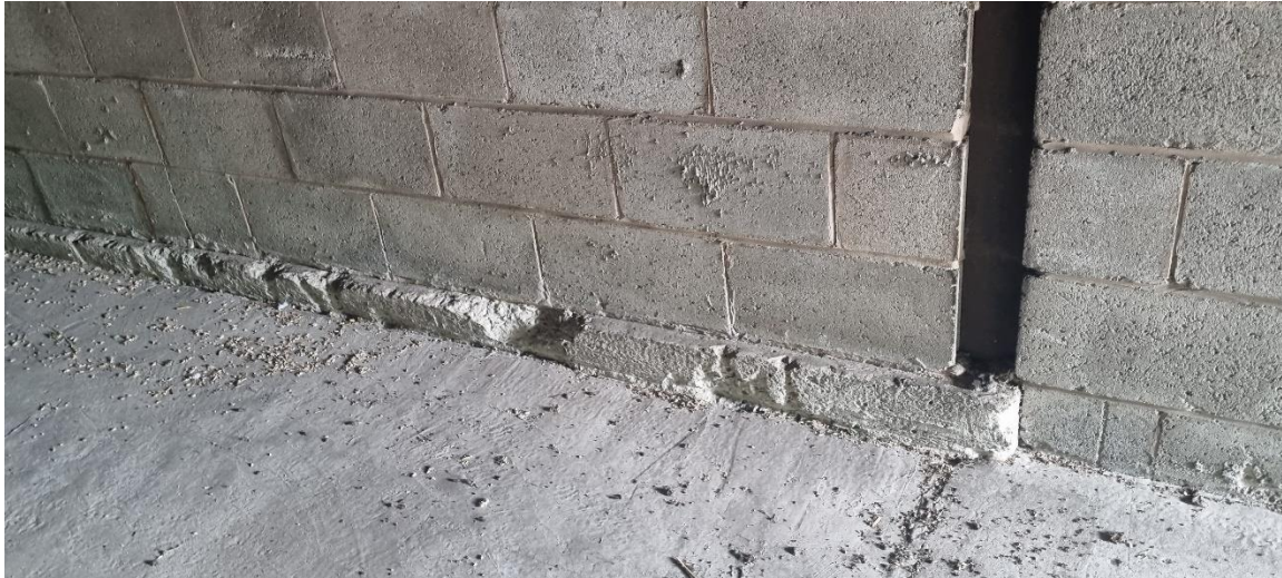
(Foam filler – gaps in the blockwork – vermin issues)
