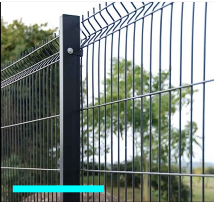
Fence Type 2 - Steel Mesh Fencing 4.2m high steel mesh fence.
