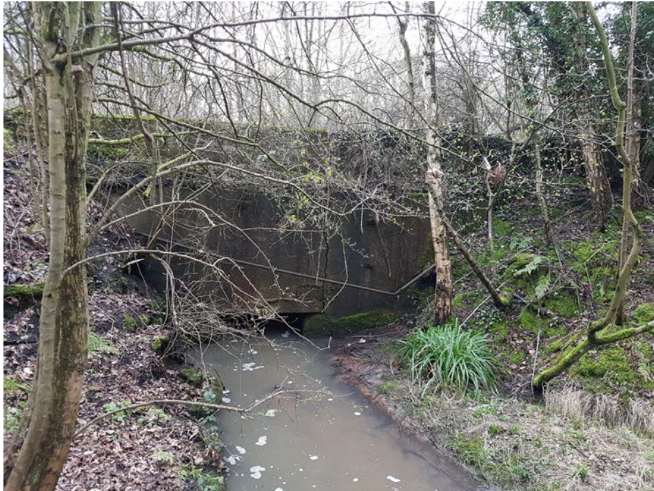
Photograph 5: Bridge/embankment structure with vertical crack along the line of the potential southern access road.
