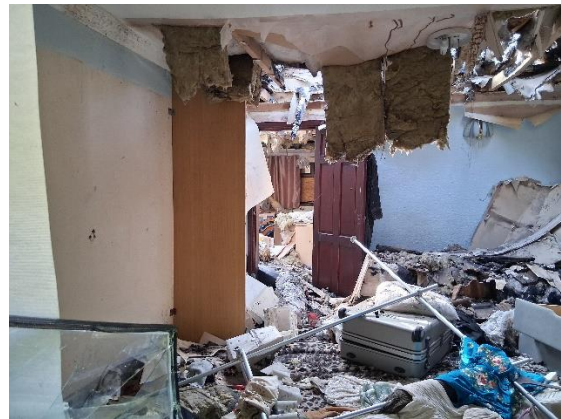
Photo 2. Internal photos of ground floor of Building 1. Open to elements.
