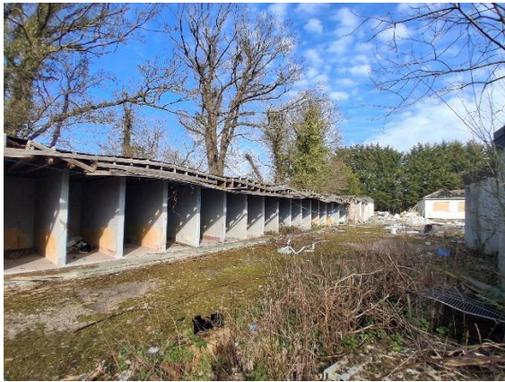
Photo 3. Building 2. Former kennels in dilapidated condition.
