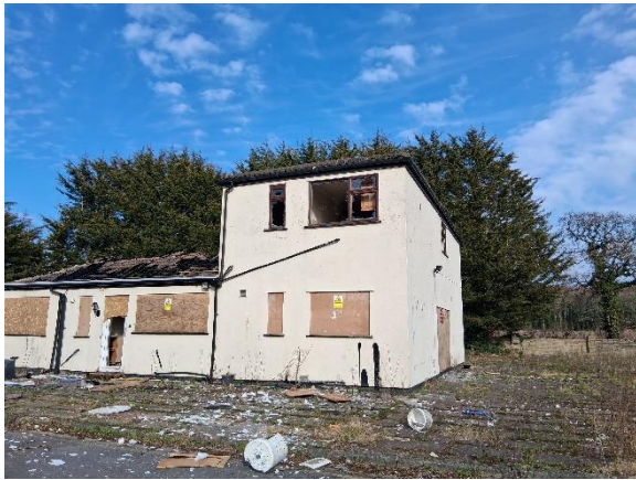
Photo 1. Building 1. Former residential property. Subject of arson (roof of single storey destroyed and main roof opened to the north / ceiling partially collapsed).
