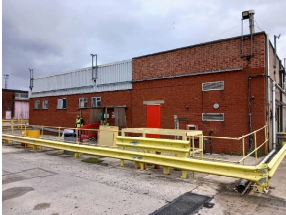
Photograph 1 – B1: Multiple gaps in brickwork and around ducting on north and east aspect. Gaps in brick under roofline. Gaps under metal cladding on north, south and west aspects.
