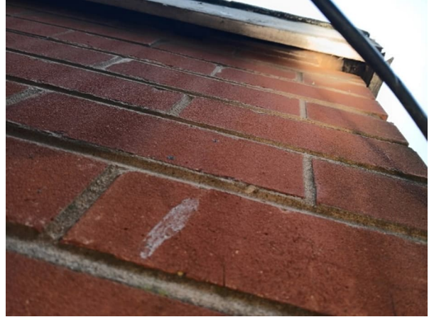
Photograph 2 – B2: Missing bricks in gap under roof on all 4 corners of building.
