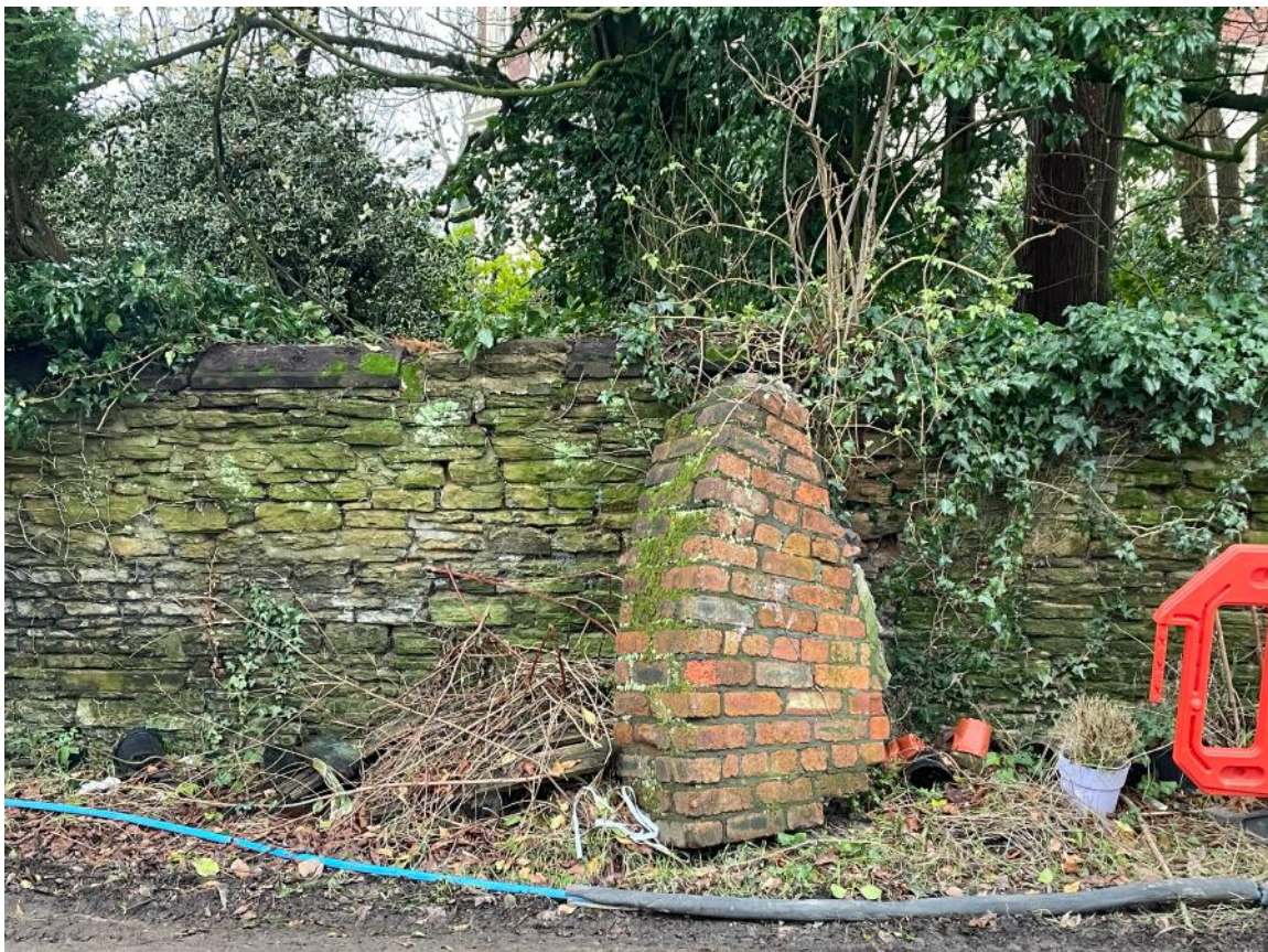
Photo 4: North Side of Wall - Broken Buttress
