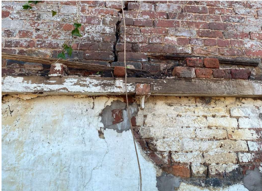
Plate 4 – Remaining timber and metal bracket to be removed.
