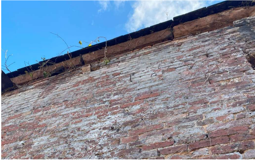
Plate 6 – Red stone blocks to be re-bed to the northwest rear elevation.
