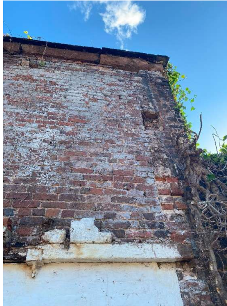
Plate 3 – Typical example of damaged bricks where brickwork replacement is proposed
