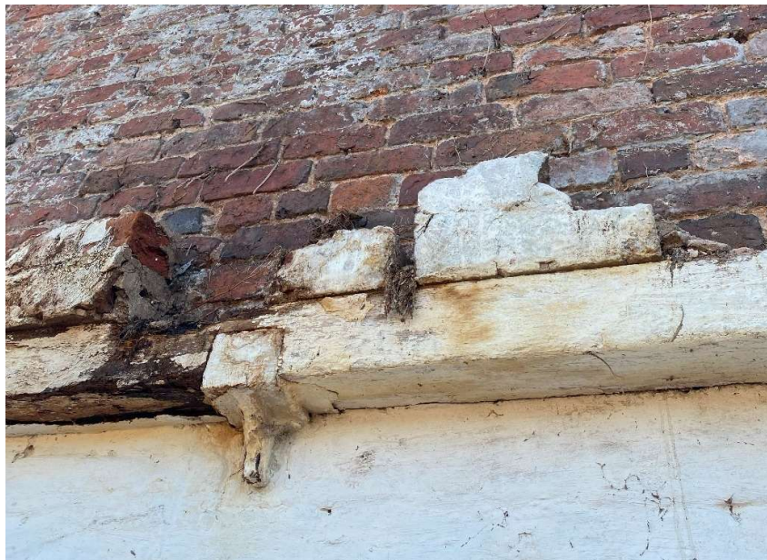
Plate 5 – Remaining timber and metal bracket to be removed.
