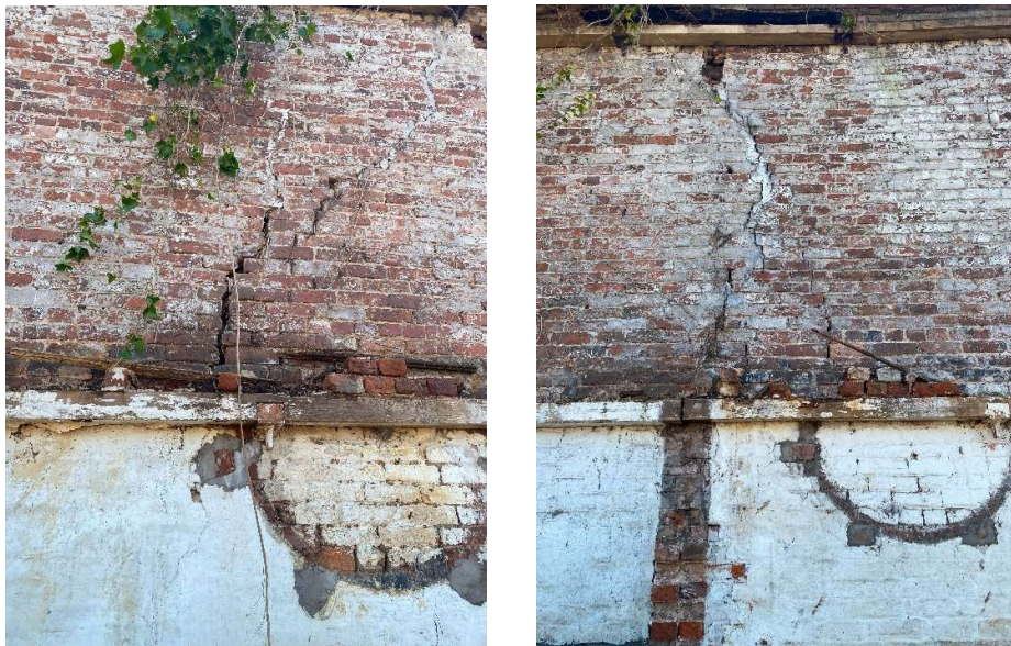
Plates 1 and 2 - Vertical cracking exposed to the first floor of the north elevation.
