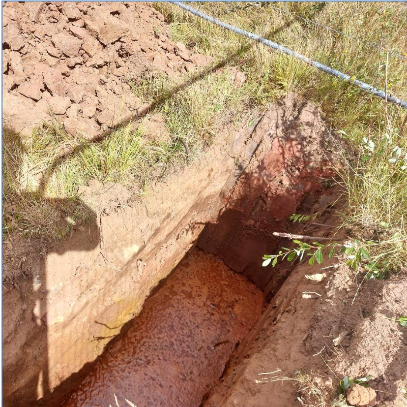
Photo 2: Compacted red clay subsoil near observation point 3 (see Map 1)
