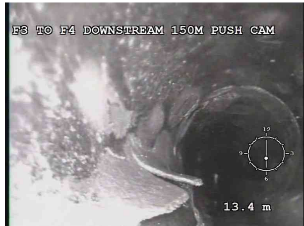
2, 00:01:07, 13.40 m Fracture, circumferential from 7 o'clock to 8 o'clock
