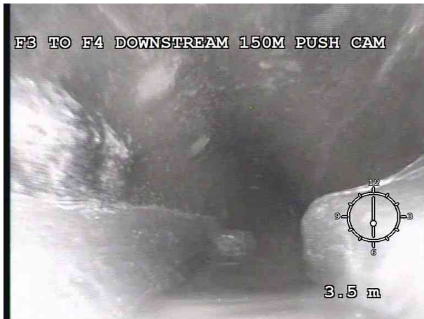
1, 00:00:22, 3.50 m General photograph taken at this point, Blisters in pipe
