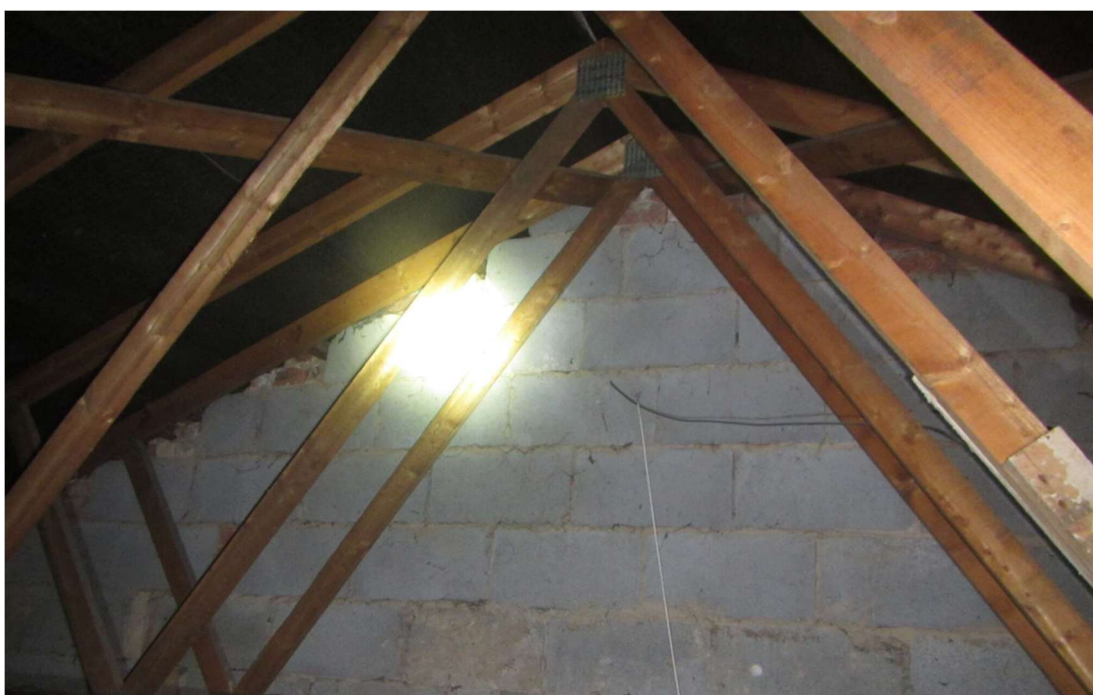
Photograph 24 – Gaps above the wall plate within the loft space of Building 7.
