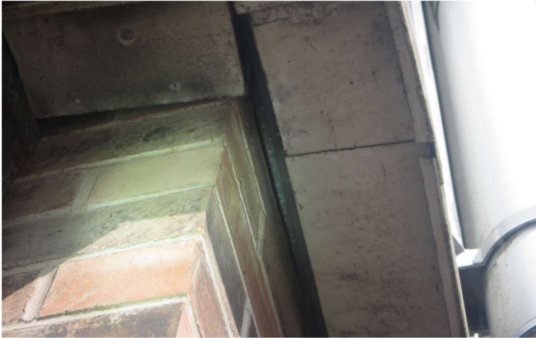
Photograph 7 – A gap between the eaves and external wall on Building 1.
