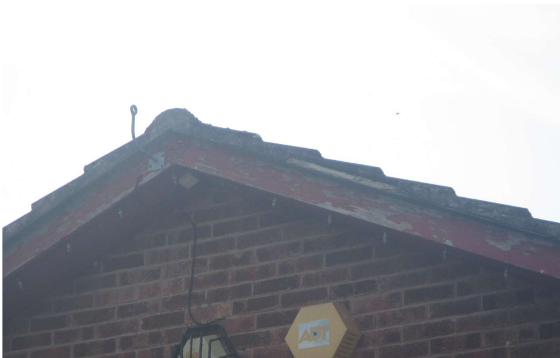
Photograph 16 – Missing mortar in the verge pointing of Building 7.
