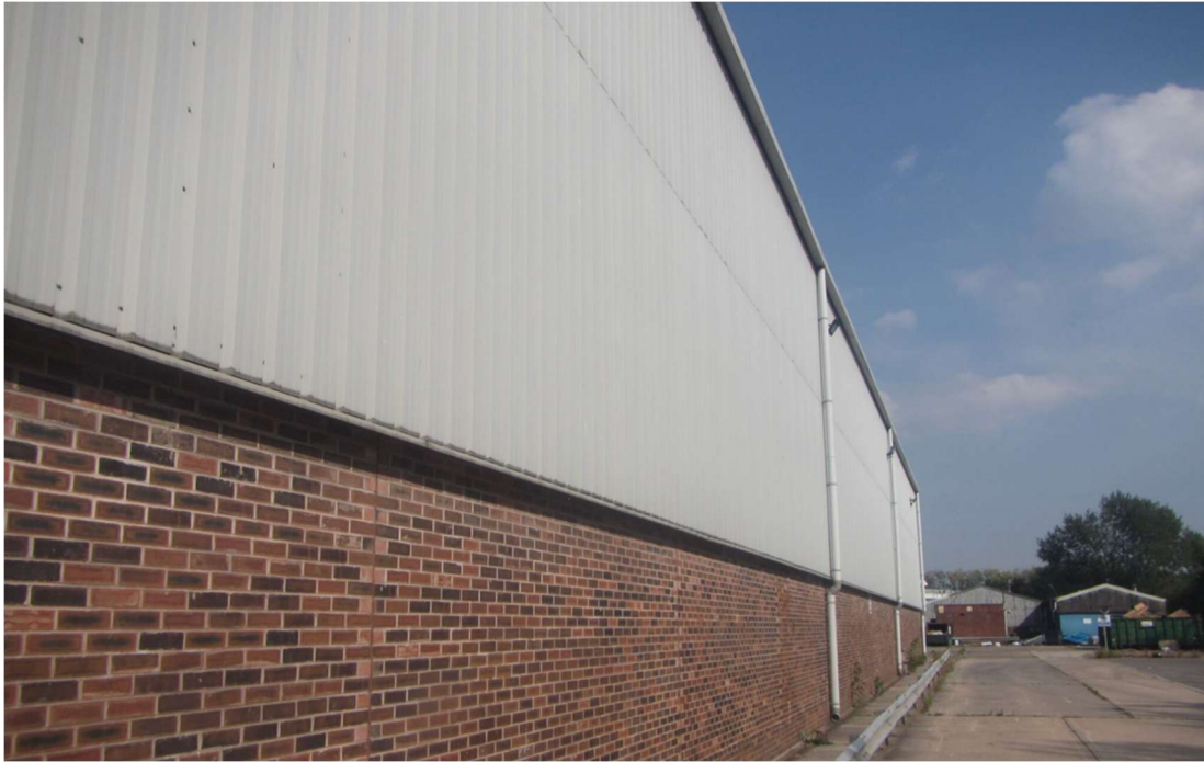
Photograph 9 – Gaps are present underneath the metal cladding and external walls on Building 1.
