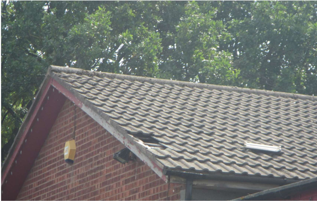
Photograph 17 – Missing tiles on the roof of Building 7.
