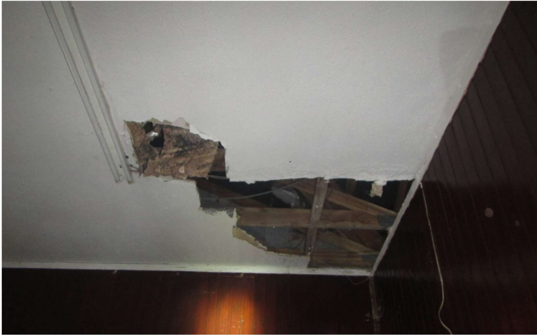
Photograph 21 – A damaged false ceiling within Building 7.
