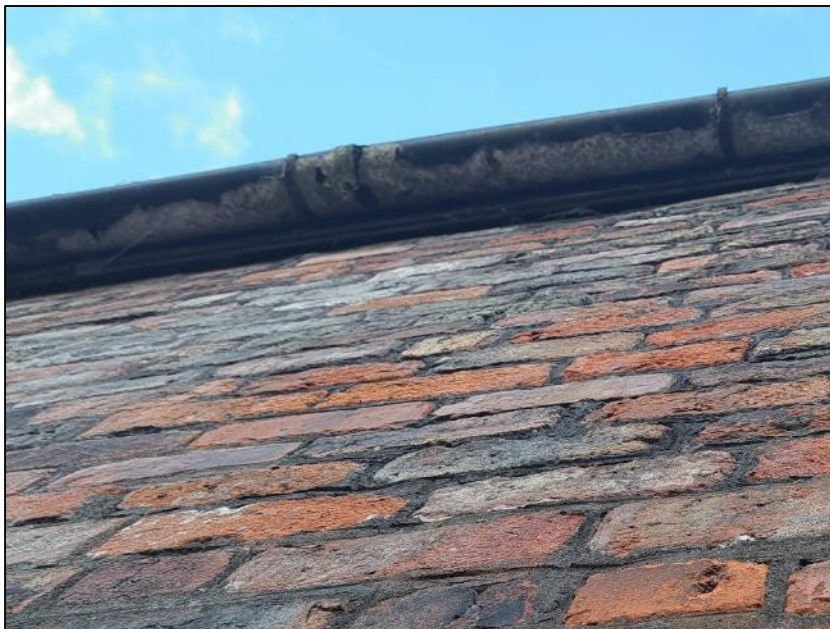
Photograph 13 showing gaps under the fascia
