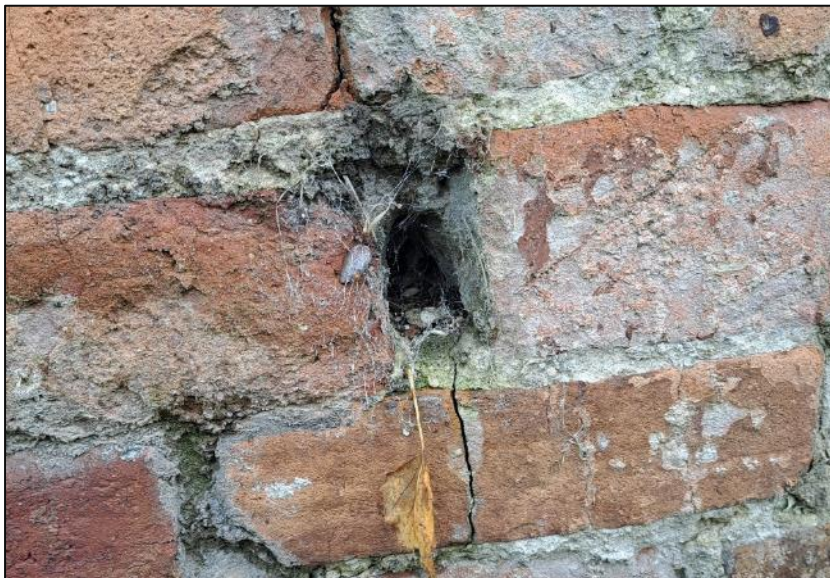
Photograph 17 showing a cavity in the wall
