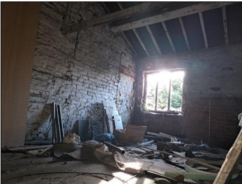
Photograph 21 showing the upper elevation of the western section of the barn and smashed window
