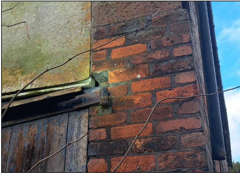
Photograph 12 showing gaps in the external brickwork
