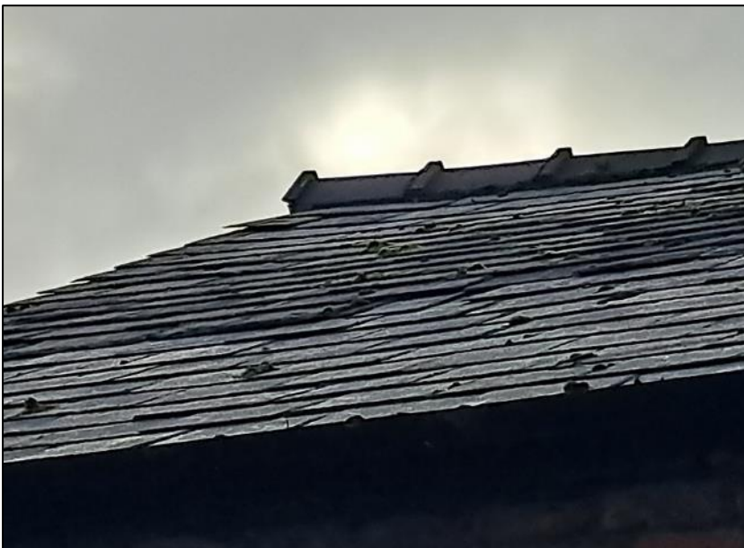
Photograph 15 showing lifted tiles
