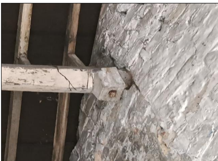
Photograph 23 showing cavities in the brickwork
