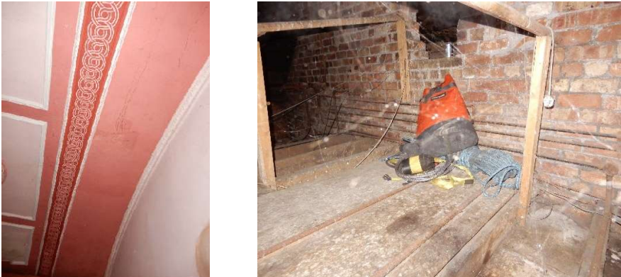
Photos 58 & 59: The partial small 7 th bay which is 800 mm wider at its western end. The plaster at its apex is damaged; From above it is clear that this damage has been caused by people using the main access point above.
