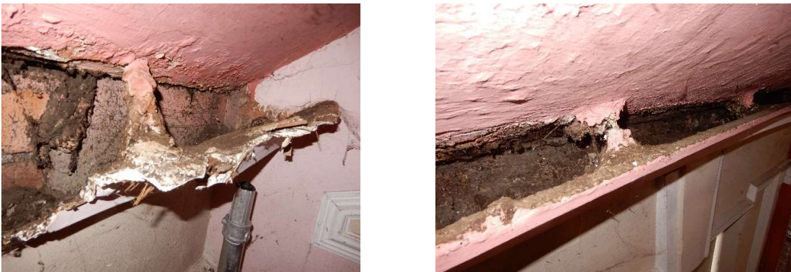
Photos 74-75: With also failing wads trying to support a water damaged and warped cornice below
