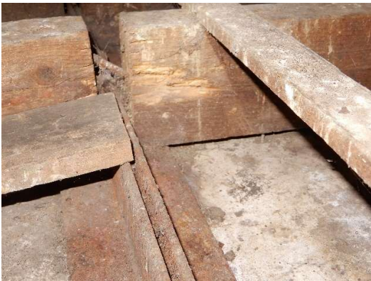
Photo 9: Whilst generally the ceiling joists are in good condition there are some localised signs of rot and occasionally a lack of bearing on the lower members of the trusses.
