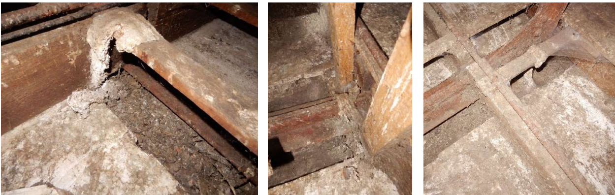
Photos 72-73: The few remaining plaster and hessian only nibs have deteriorated and snapped.
