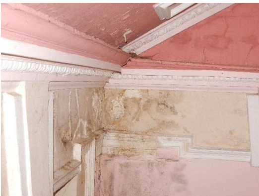
Photo 30: Excessive water damaged ceiling and wall plaster can be found at the eastern end of the first bay
