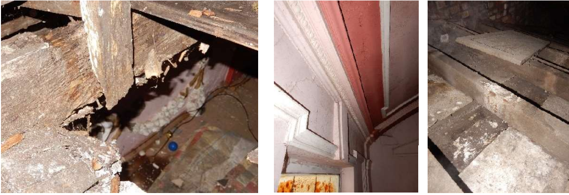
Photos 55-57: The rotten timbers above the western third of the 6 th bay; the cracked and de-bonded wall plaster on the wall; and the missing plaster wads that should be holding the rib up between the 6 th and 7 th bay.
