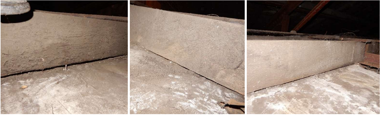
Photos 69-71: Many of the cast panels are warped and some are pulling off the bottom of the ceiling joists which they are nailed on to.
