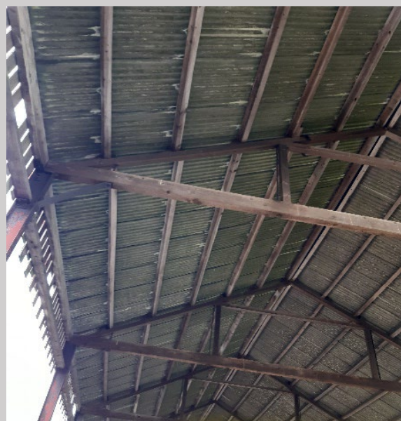
Photograph 14: Main Barn unlined roof
