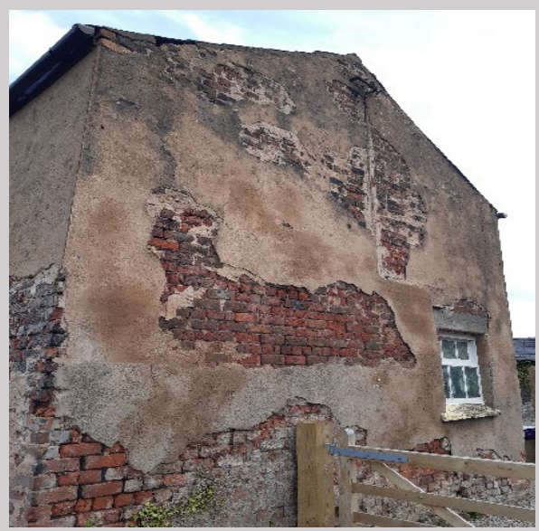
Photograph 10: Stone Barn B red bricks and damaged render (western aspect)
