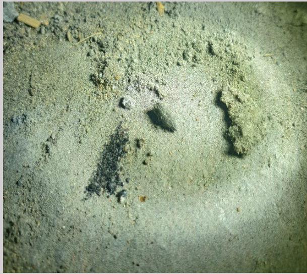
Photograph 17: Bat droppings found within the Piggery on half-height internal wall
