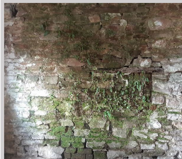
Photograph 11: Stone Barn A – B adjoining wall damage
