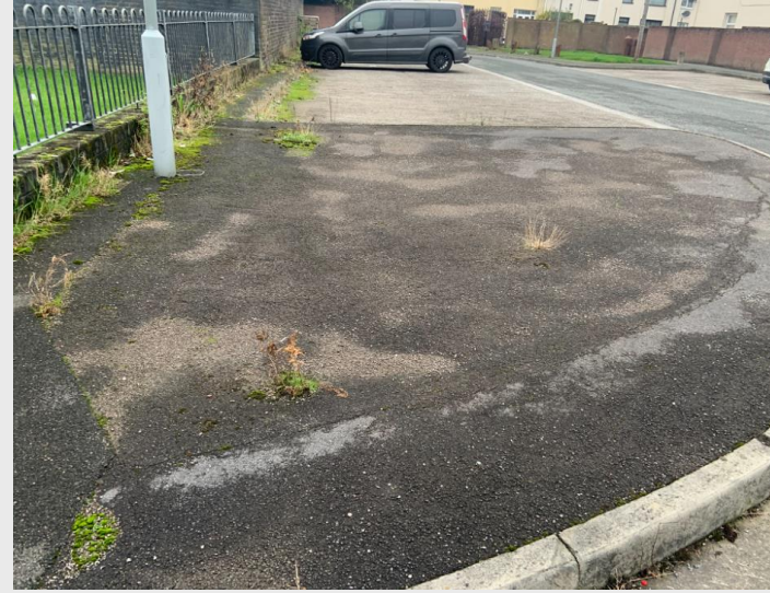
Photograph 6: View of a raised area of pavement.
