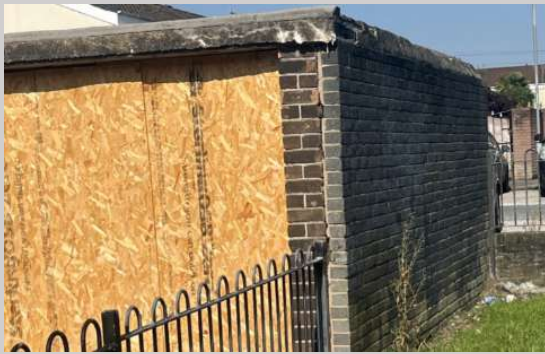
Photograph 3: Sealed garage entrance with small crack visible along the exterior wall next to metal fencing.
