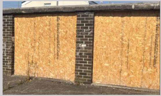
Photograph 2: Fully sealed garage doors with plywood cover.
