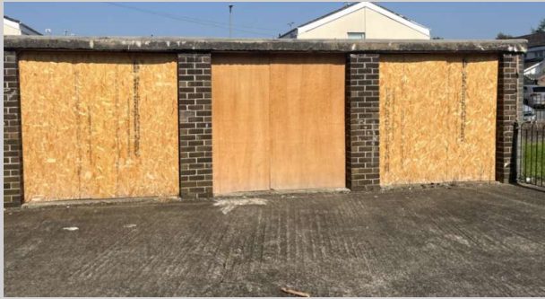
Photograph 1: Fully sealed garage doors with plywood cover.
