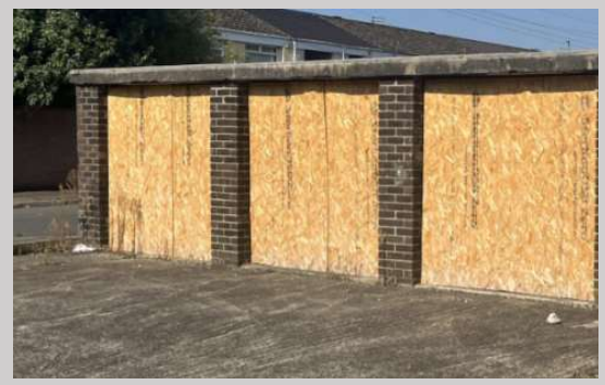
Photograph 4: Remaining garage entrances, sealed roof and no overhang or fascias.
