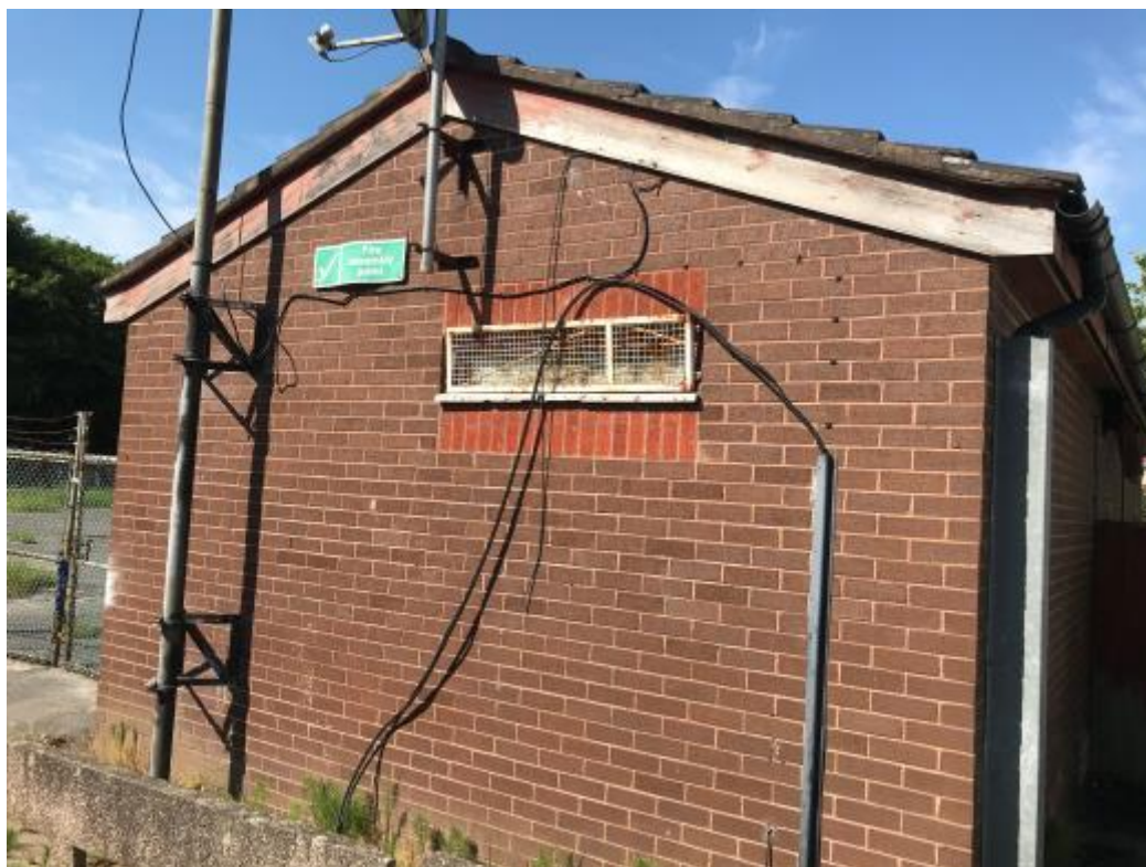
Plate 2 – The eastern elevation of the outbuilding, with gaps between the window cover
