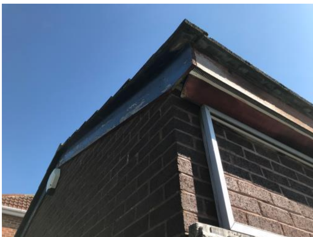
Plate 6 – Minor gap in the soffit box
