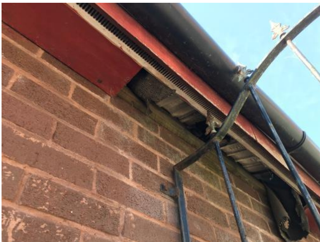
Plate 5 – Major gap in the broken soffit
