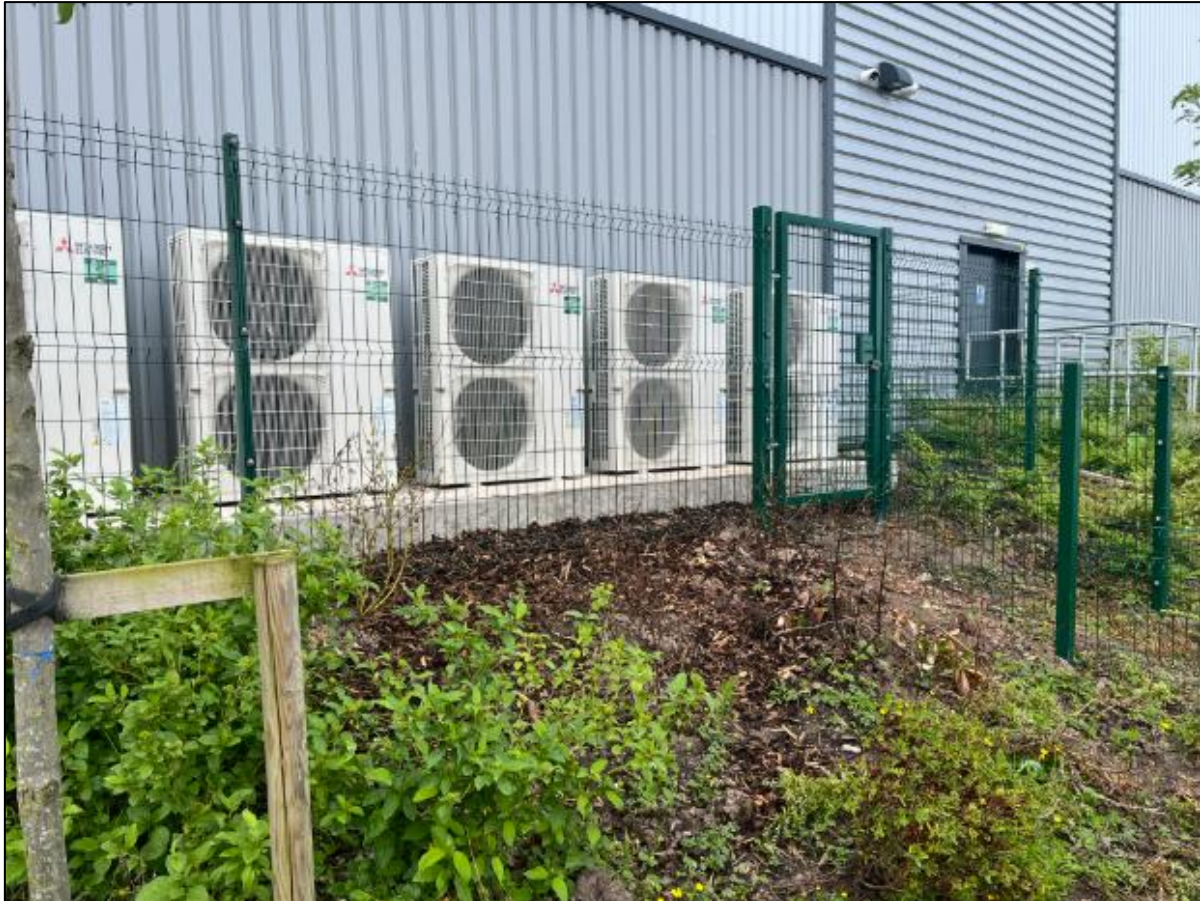
Figure 5.1 – Imagery taken during site visit on 5 th June 2026 indicating placement of AC units in place of vegetation.
