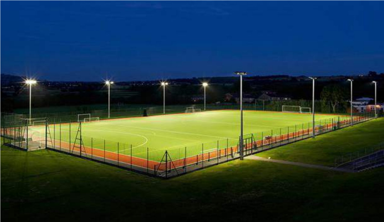
Column mounted floodlights
