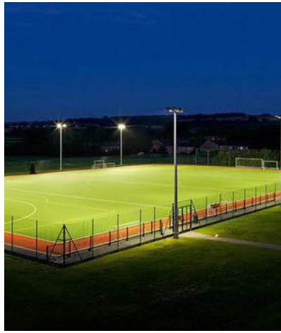
Floodlighting at football pitches
