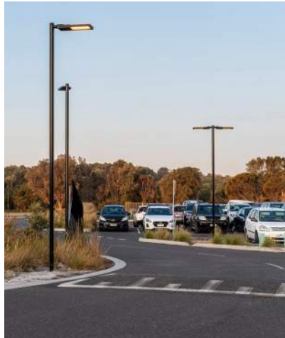
Column lighting for car park
