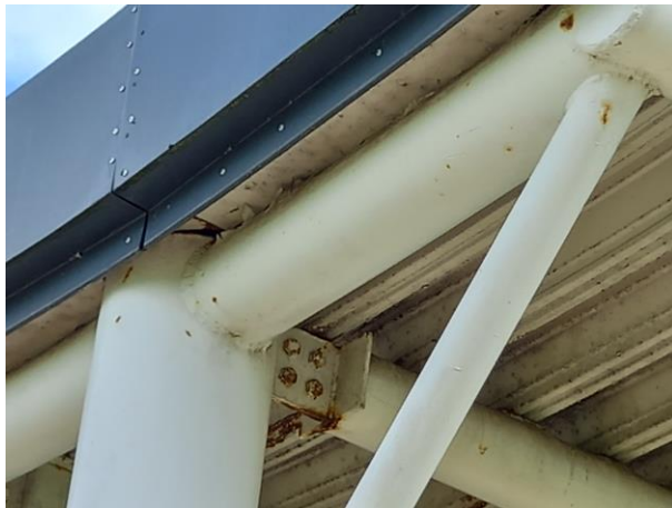
Photograph 17 – Halewood leisure centre potential bat roost feature (PRF), gaps in soffit where support post meets the building canopy.
