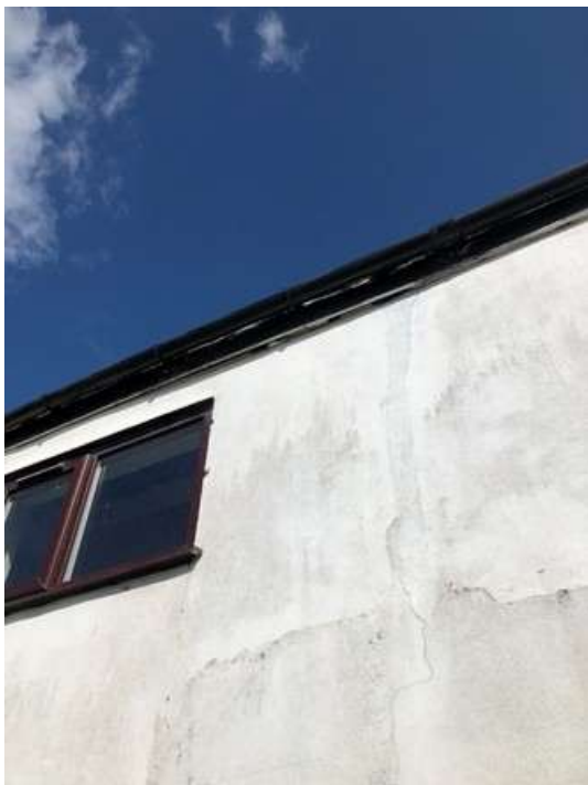
Photo 3: Lifted barge board on western elevation of Building 1.
