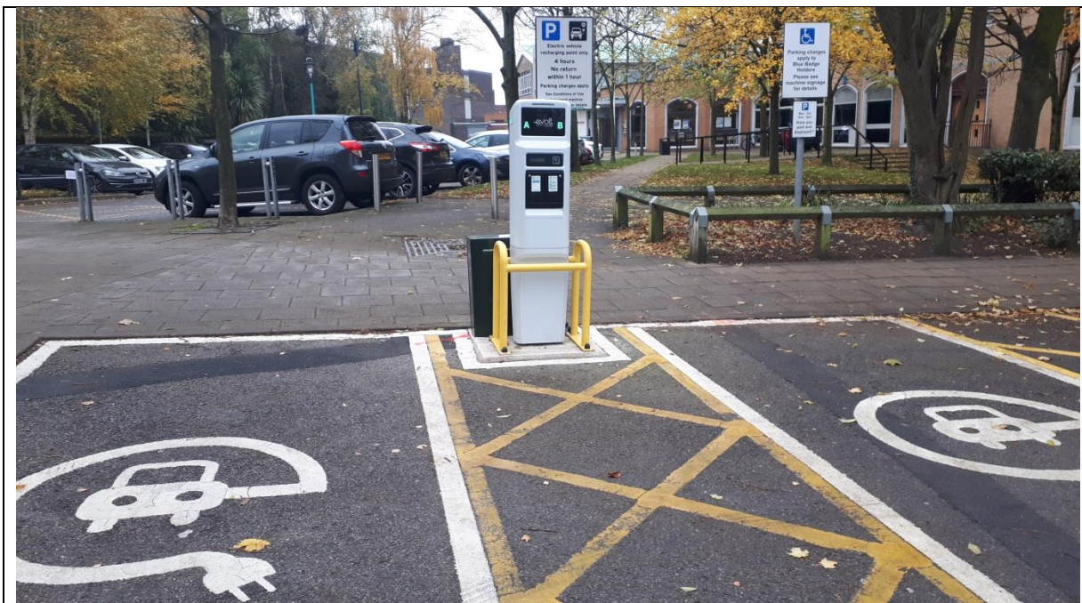
Photo 43 – Electric car charging station located on site
