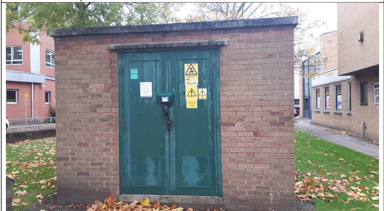
Photo 16 – Electricity Substation located on site to the south
