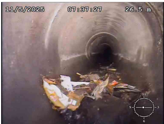
7, 00:03:44, 26.50 m Settled deposits, coarse, 5% cross-sectional area loss, start
