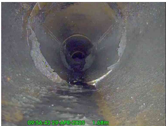
3, 00:00:14, 1.68 m Roots, mass at joint, 5% cross-sectional area loss
