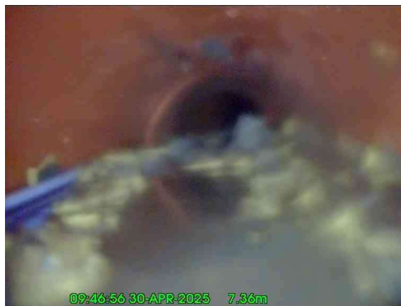
6, 00:01:58, 7.36 m Settled deposits, hard or compacted, 25% cross-sectional area loss, change, Solid set debris remained in sewer following jetting
