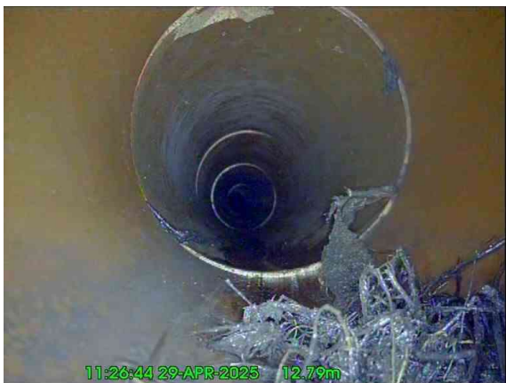
11, 00:01:01, 12.79 m Surface damage, increased roughness from 11 o'clock to 12 o'clock
