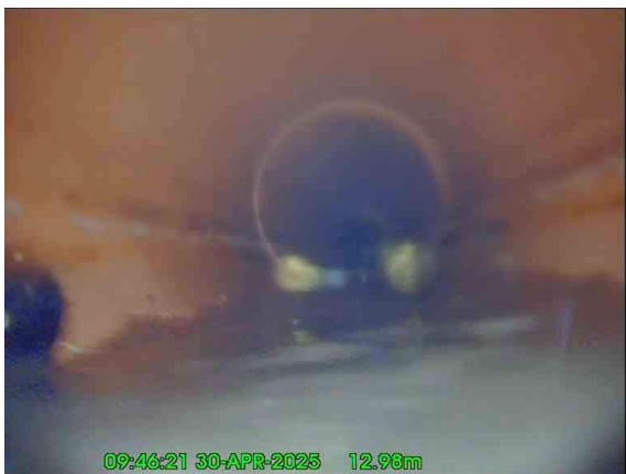
7, 00:01:23, 12.98 m Settled deposits, hard or compacted, 25% cross-sectional area loss, finish, Solid set debris remained in sewer following jetting
