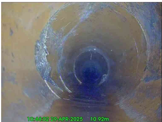
9, 00:01:20, 10.92 m Roots, mass at joint, 5% cross-sectional area loss
