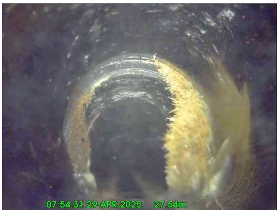
7, 00:02:06, 27.54 m Roots, mass at joint, 20% cross-sectional area loss
