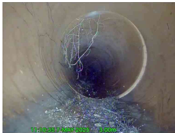
2, 00:00:20, 3.00 m Roots, mass at joint, 5% cross-sectional area loss
