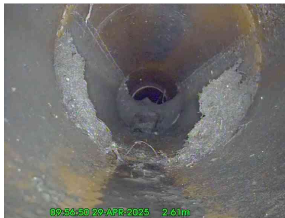
4, 00:00:21, 2.61 m Roots, mass at joint, 10% cross-sectional area loss
