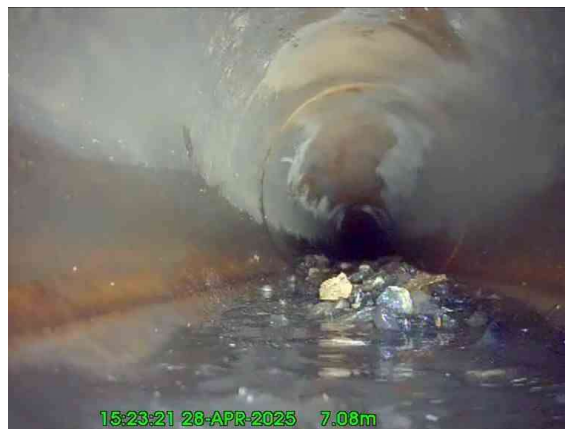
2, 00:05:12, 7.08 m Settled deposits, coarse, 5% cross-sectional area loss, start
