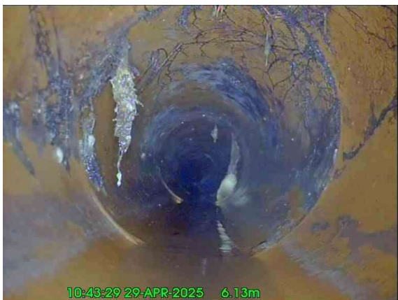
5, 00:00:47, 6.13 m Roots, mass at joint, 5% cross-sectional area loss
