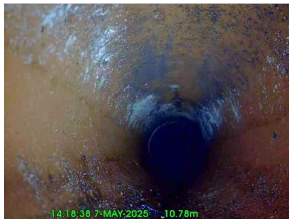
6, 00:00:52, 10.78 m Settled deposits, fine, 10% cross-sectional area loss, finish
