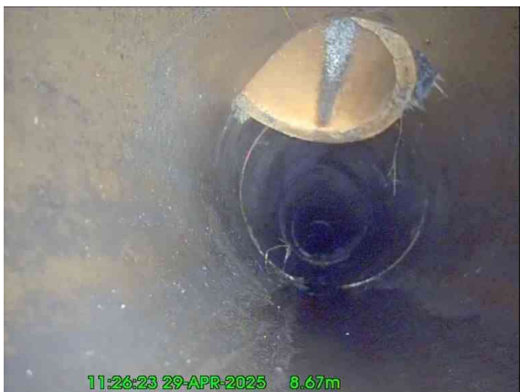
5, 00:00:41, 8.67 m Connection defective, connecting pipe is intruding at 12 o'clock, 100mm dia, intrusion: 20%
