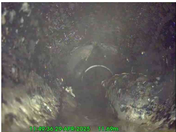
5, 00:01:44, 11.69 m Deformed sewer or drain, 20%
