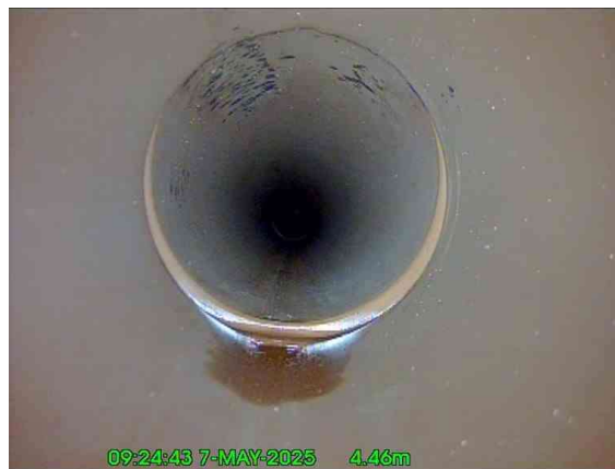
2, 00:00:19, 4.46 m Joint displaced, medium
