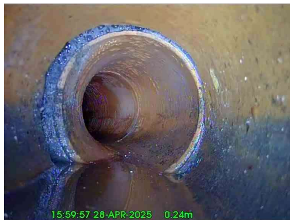
2, 00:00:05, 0.24 m Joint displaced, medium
