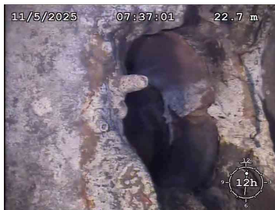
6, 00:03:18, 22.70 m Connection other than junction at 11 o'clock, 150mm dia
