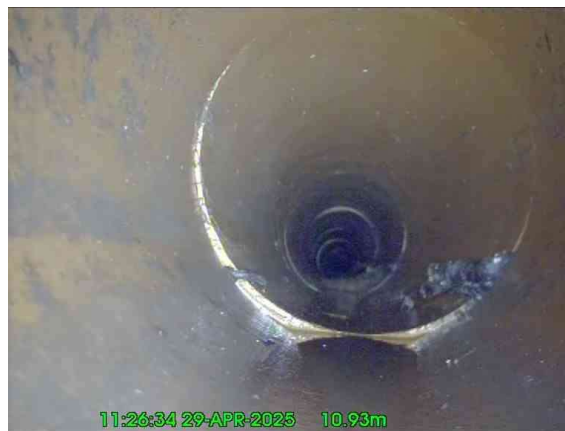
8, 00:00:52, 10.93 m Roots, tap at joint
