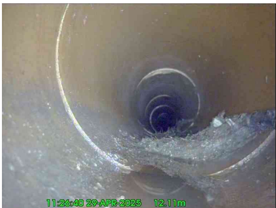
9, 00:00:57, 12.11 m Roots, mass at joint, 5% cross-sectional area loss
