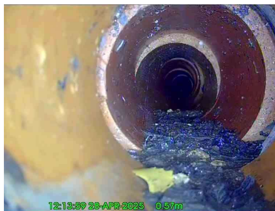
4, 00:00:14, 0.57 m Settled deposits, fine, 5% cross-sectional area loss
