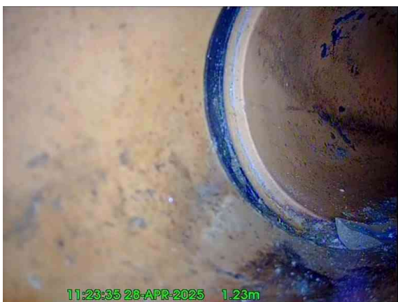
3, 00:00:19, 1.23 m Joint displaced, medium
