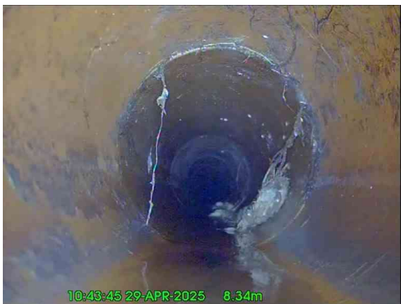
7, 00:01:03, 8.34 m Roots, mass at joint, 5% cross-sectional area loss
