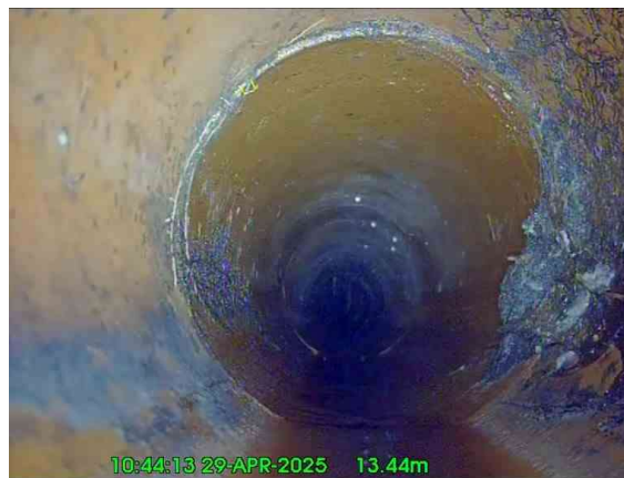
12, 00:01:31, 13.44 m Roots, mass at joint, 5% cross-sectional area loss
