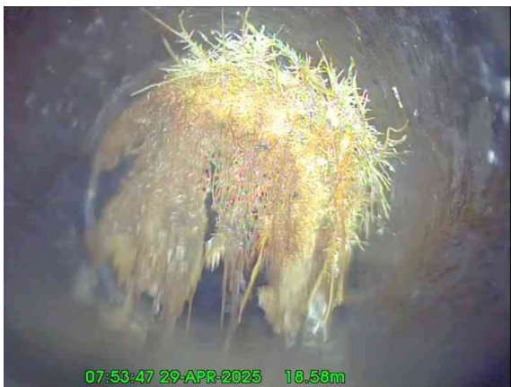
3, 00:01:21, 18.58 m Roots, mass at joint, 75% cross-sectional area loss
