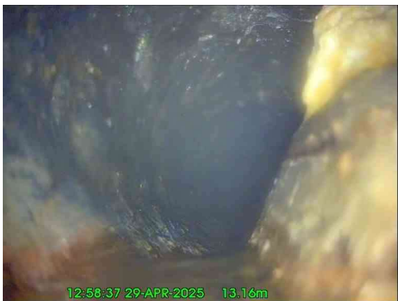
3, 00:02:29, 13.16 m Deformed sewer or drain, 25%
