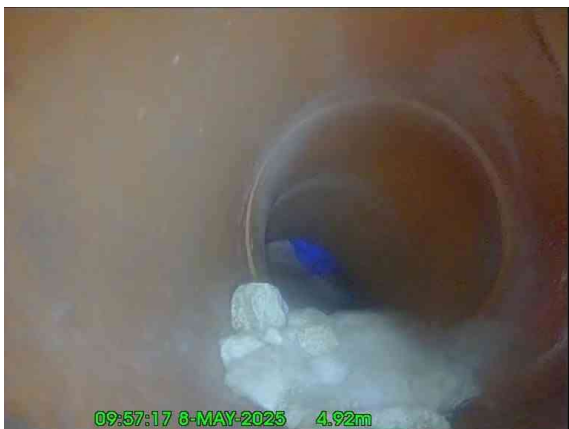
5, 00:00:23, 4.92 m Settled deposits, coarse, 10% cross-sectional area loss
