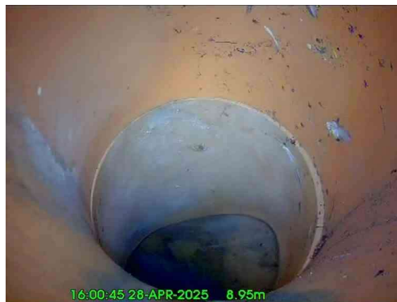
6, 00:00:53, 8.95 m Line deviates down
