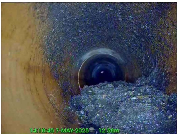
7, 00:01:00, 12.58 m Settled deposits, fine, 20% cross-sectional area loss
