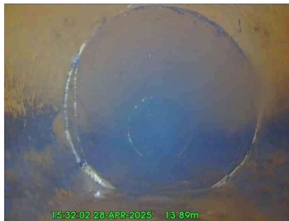
4, 00:01:03, 13.89 m Crack, circumferential at joint from 8 o'clock to 10 o'clock
