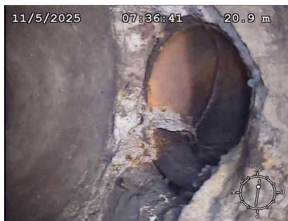
4, 00:02:58, 20.90 m Connection other than junction at 1 o'clock, 150mm dia
