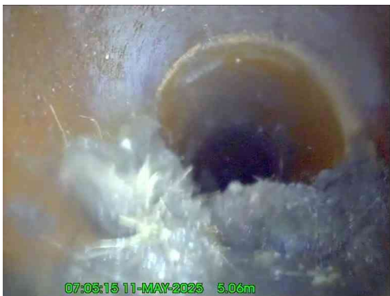
3, 00:00:22, 5.06 m Roots, mass at joint, 25% cross-sectional area loss
