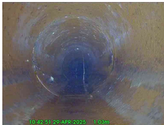
2, 00:00:08, 1.03 m Roots, fine at joint
