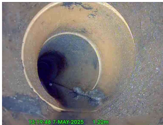
2, 00:00:07, 1.22 m Line deviates left
