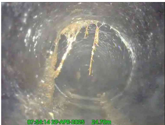
5, 00:01:48, 24.70 m Roots, mass at joint, 5% cross-sectional area loss
