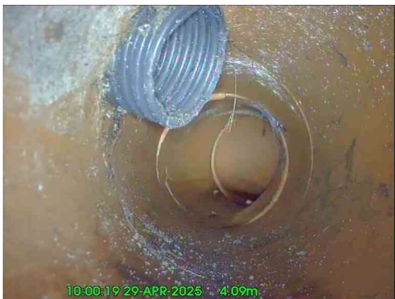
3, 00:00:36, 4.09 m Connection defective, connecting pipe is intruding at 10 o'clock, 100mm dia, intrusion: 20%
