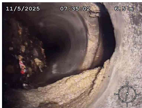
2, 00:01:19, 6.50 m Connection other than junction at 2 o'clock, 150mm dia
