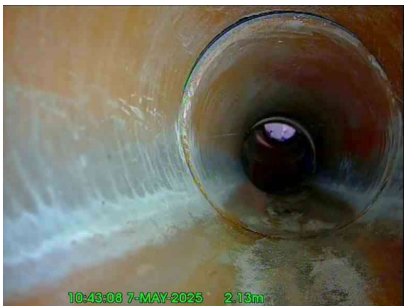
3, 00:00:20, 2.13 m Joint displaced, medium
