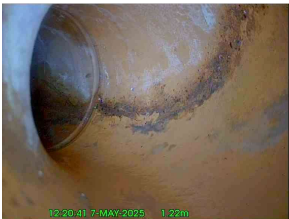
3, 00:00:15, 1.22 m Line deviates left
