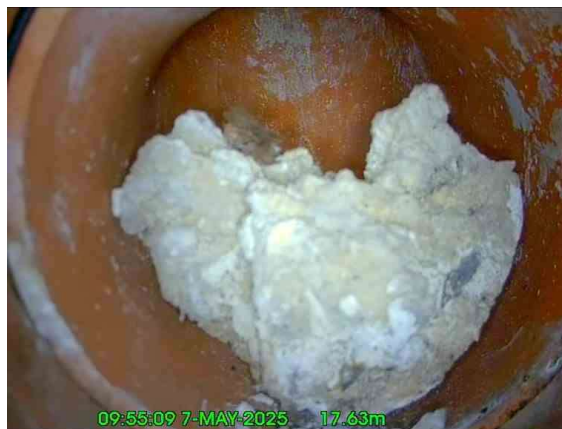
6, 00:01:48, 17.63 m Settled deposits, hard or compacted, 35% cross-sectional area loss, Unable to remove solid set debris via jetting
