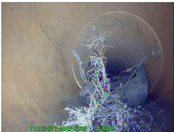
3, 00:00:27, 4.84 m Roots, mass at joint, 10% cross-sectional area loss
