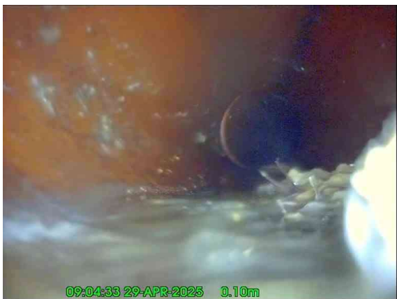
1, 00:02:45, 0.10 m Roots, mass at joint, 10% cross-sectional area loss
