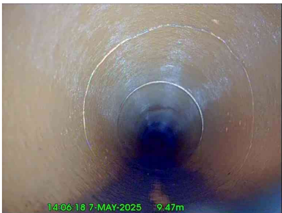
3, 00:00:34, 9.47 m Crack, circumferential from 8 o'clock to 4 o'clock
