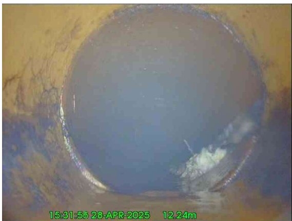
3, 00:00:52, 12.24 m Roots, mass at joint, 5% cross-sectional area loss
