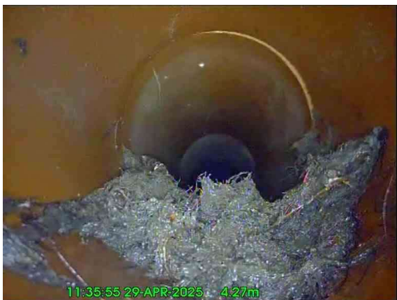
3, 00:02:57, 4.27 m Roots, mass at joint, 20% cross-sectional area loss, change
