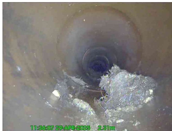
2, 00:03:09, 2.31 m Roots, mass at joint, 10% cross-sectional area loss, start
