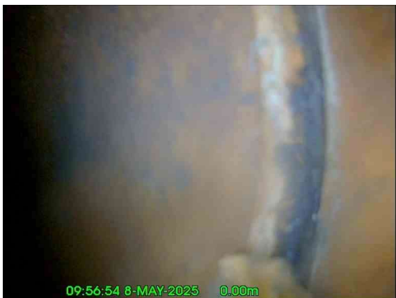
1, 00:00:02, 0.00 m Line deviates left
