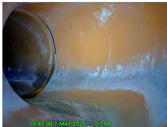
2, 00:00:12, 0.75 m Line deviates left
