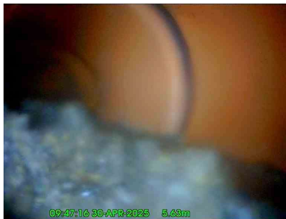
4, 00:02:18, 5.63 m Joint displaced, medium
