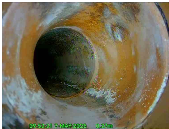
2, 00:00:10, 0.37 m Line deviates left
