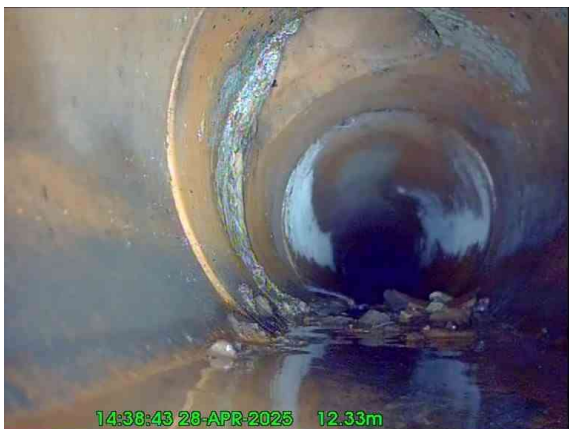
5, 00:01:09, 12.33 m Settled deposits, coarse, 5% cross-sectional area loss, start
