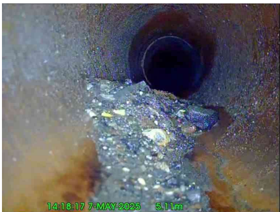
3, 00:00:31, 5.11 m Settled deposits, fine, 10% cross-sectional area loss
