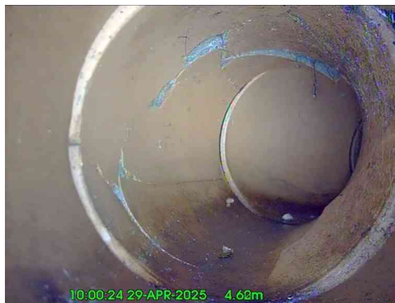
4, 00:00:41, 4.62 m Fractures, multiple at joint from 7 o'clock to 1 o'clock
