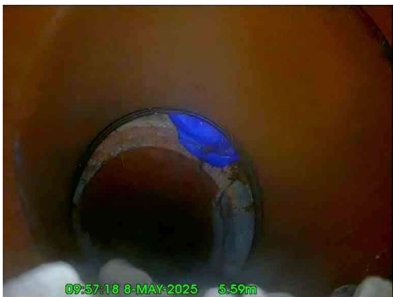
7, 00:00:24, 5.59 m Joint displaced, large
