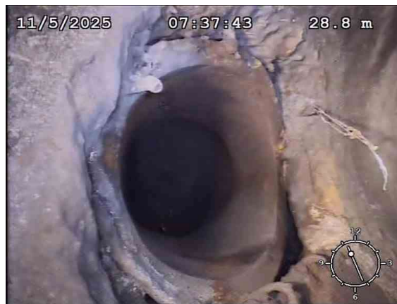
8, 00:04:00, 28.80 m Connection other than junction at 11 o'clock, 150mm dia
