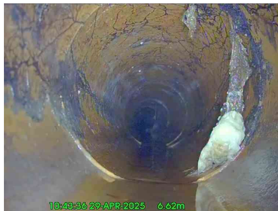
6, 00:00:54, 6.62 m Roots, mass at joint, 5% cross-sectional area loss
