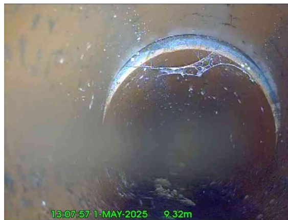
4, 00:00:50, 9.32 m Joint displaced, medium
