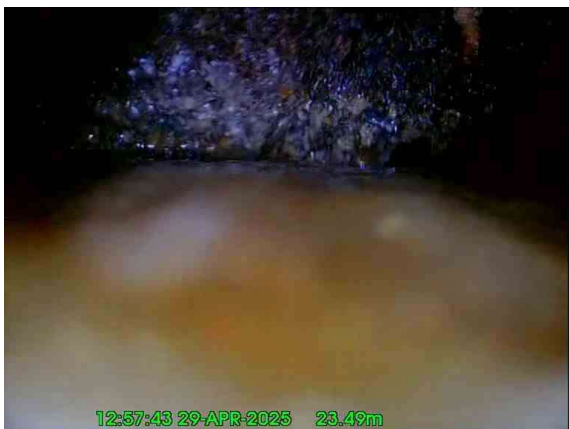
9, 00:01:34, 23.49 m Roots, mass, 75% cross-sectional area loss, At entry to MH20 UTL
