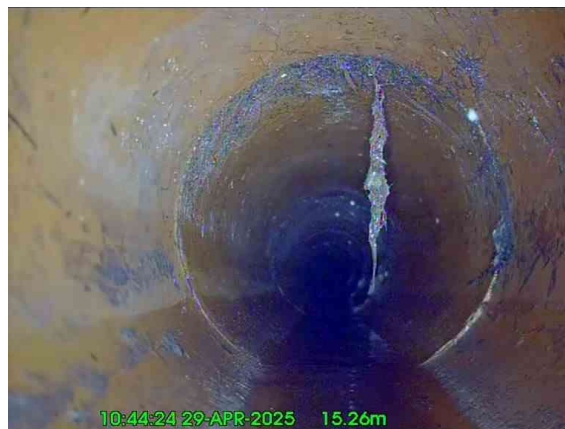
14, 00:01:42, 15.26 m Roots, fine at joint
