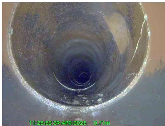
2, 00:00:09, 0.71 m Crack, circumferential at joint from 2 o'clock to 4 o'clock
