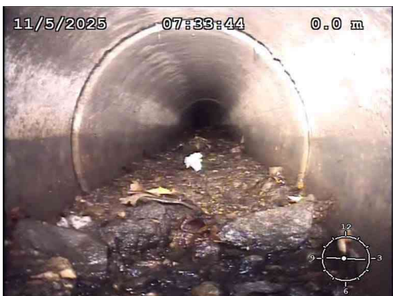
1, 00:00:01, 0.00 m Settled deposits, coarse, 20% cross-sectional area loss, start
