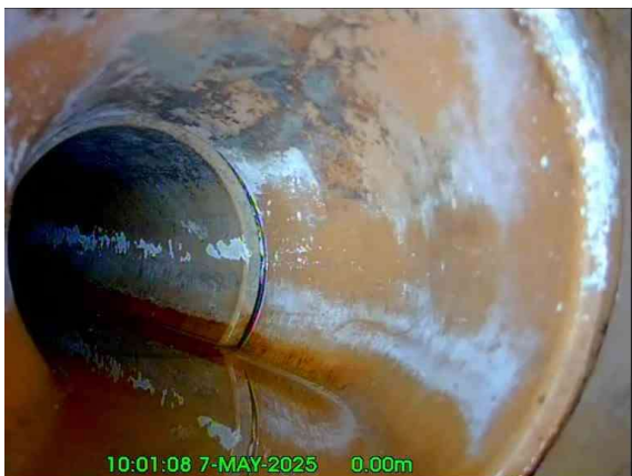
1, 00:00:01, 0.00 m Line deviates left
