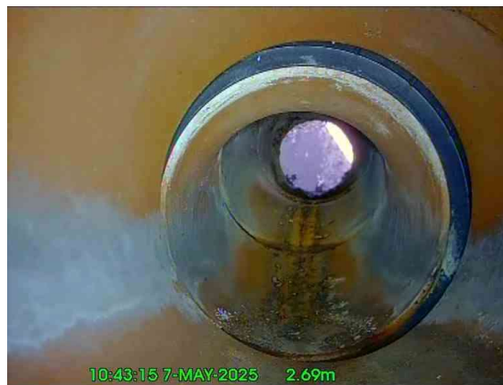
4, 00:00:27, 2.69 m Joint displaced, large
