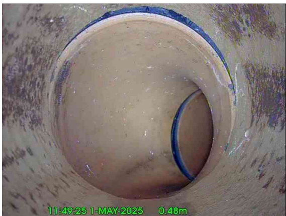
1, 00:00:10, 0.48 m Joint displaced, medium
