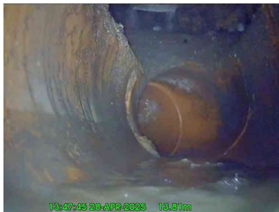
6, 00:01:37, 13.81 m Roots, mass at joint, 10% cross-sectional area loss, finish
