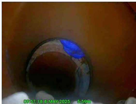
6, 00:00:24, 5.59 m Line deviates left
