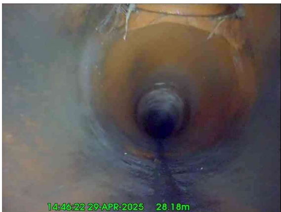
5, 00:01:07, 28.18 m Connection other than junction at 12 o'clock, 150mm dia
