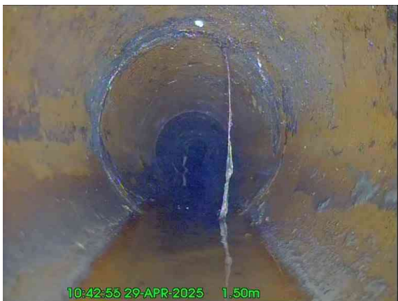
3, 00:00:13, 1.50 m Roots, fine at joint
