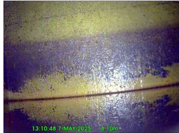
6, 00:00:02, 8.10 m Finish node, oil separator, reference: MH58 reached
