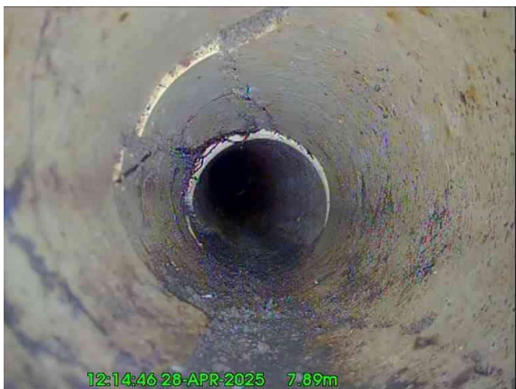
9, 00:01:01, 7.89 m Fracture, circumferential from 9 o'clock to 12 o'clock
