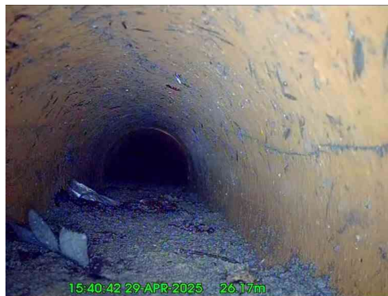
4, 00:02:12, 26.17 m Settled deposits, fine, 20% cross-sectional area loss
