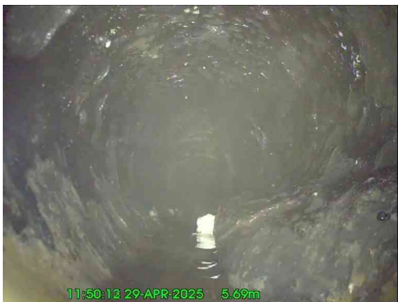
3, 00:02:21, 5.69 m Deformed sewer or drain, 5%
