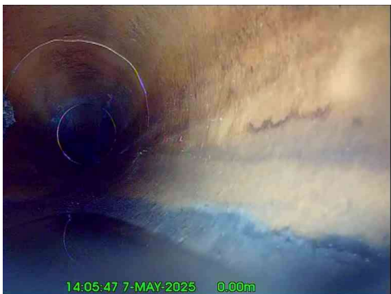
1, 00:00:02, 0.00 m Crack, circumferential from 10 o'clock to 2 o'clock
