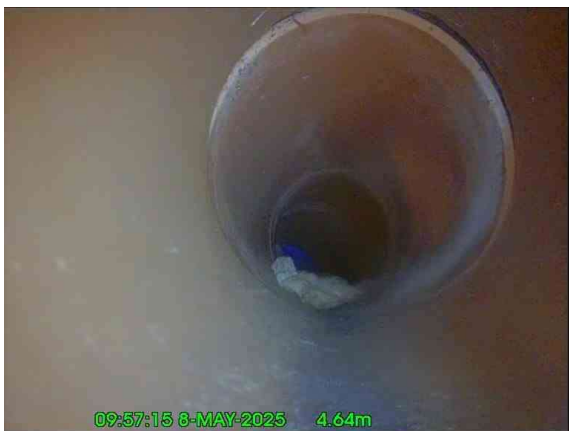
3, 00:00:22, 4.64 m Joint displaced, medium
