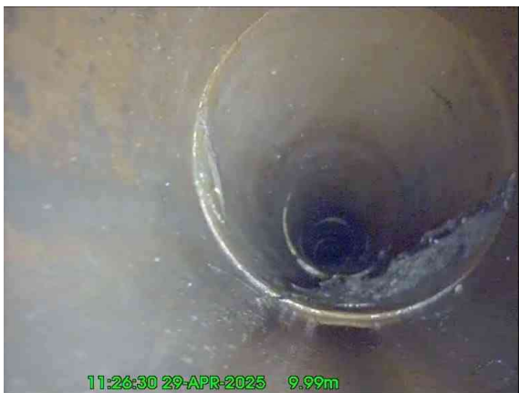
7, 00:00:48, 9.99 m Roots, mass at joint, 5% cross-sectional area loss
