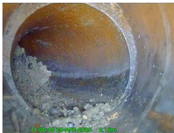
4, 00:00:33, 2.13 m Line deviates left
