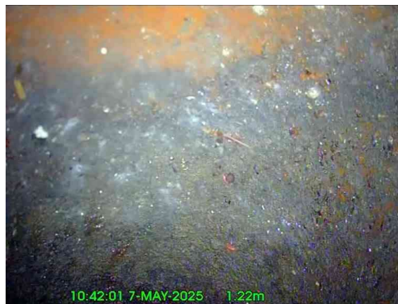
4, 00:00:16, 1.22 m Finish node, oil separator, reference: MH50 reached
