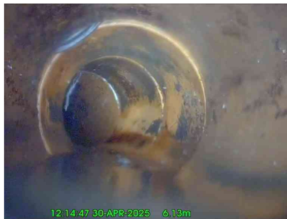
4, 00:00:32, 6.13 m Sealing ring intruding from 10 o'clock to 11 o'clock
