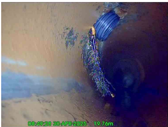
3, 00:01:24, 19.76 m Connection defective, connecting pipe is intruding at 10 o'clock, 100mm dia, intrusion: 5%
