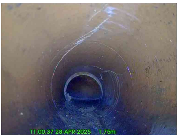
3, 00:00:30, 1.75 m Cracks, multiple at joint from 8 o'clock to 4 o'clock
