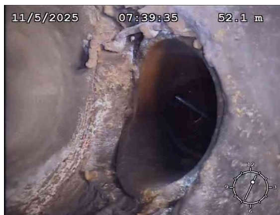
12, 00:05:52, 52.10 m Connection other than junction at 1 o'clock, 150mm dia
