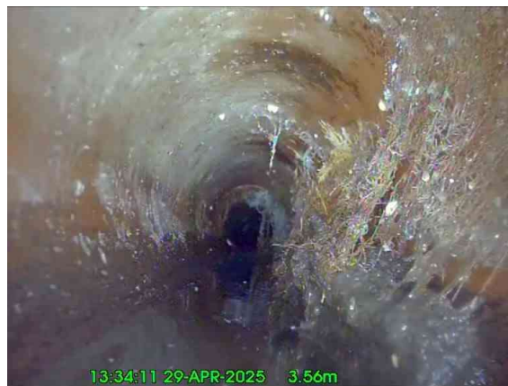
2, 00:00:25, 3.56 m Roots, mass at joint, 10% cross-sectional area loss, start
