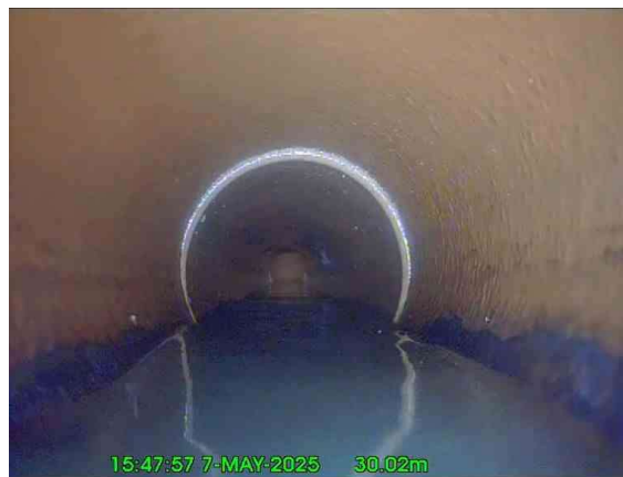
8, 00:02:47, 30.02 m Water level, 20% of the vertical dimension, Water standing in sewer
