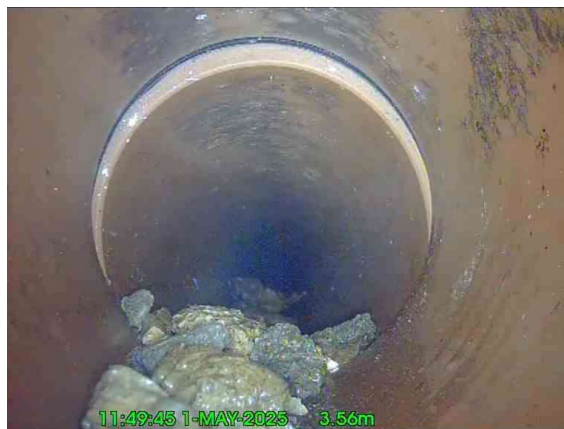
6, 00:00:30, 3.56 m Settled deposits, coarse, 5% cross-sectional area loss
