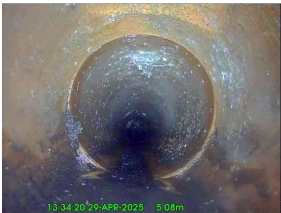
3, 00:00:34, 5.08 m Roots, mass at joint, 10% cross-sectional area loss, finish
