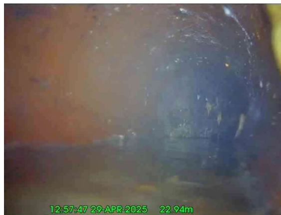
8, 00:01:39, 22.94 m Water level, 10% of the vertical dimension, Water standing in sewer due to mass roots at entry to MH20 UTL
