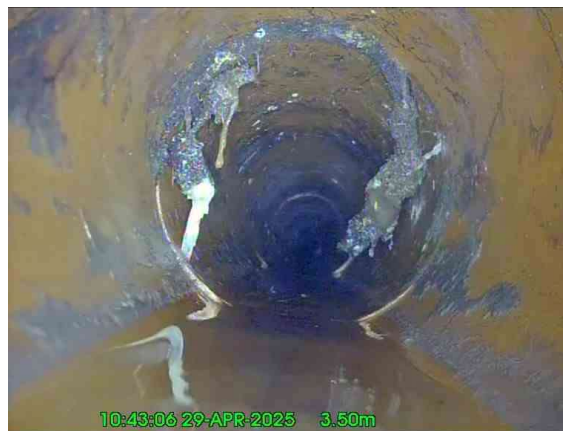
4, 00:00:24, 3.50 m Roots, mass at joint, 10% cross-sectional area loss
