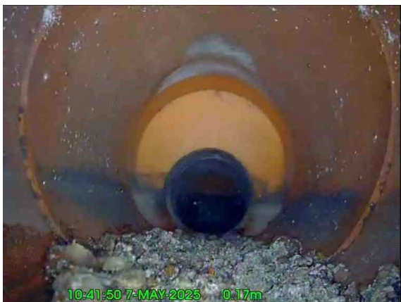
1, 00:00:05, 0.17 m Settled deposits, fine, 5% cross-sectional area loss
