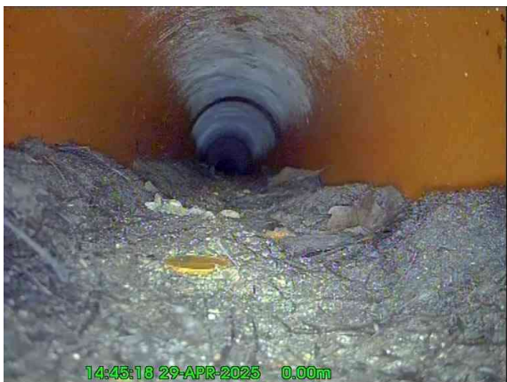
1, 00:00:03, 0.00 m Roots, mass, 20% cross-sectional area loss, start
