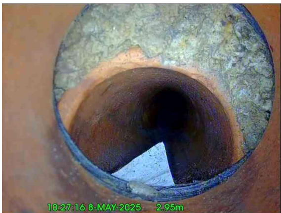
3, 00:00:14, 2.95 m Joint displaced, large
