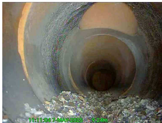
6, 00:00:49, 9.24 m Settled deposits, coarse, 5% cross-sectional area loss
