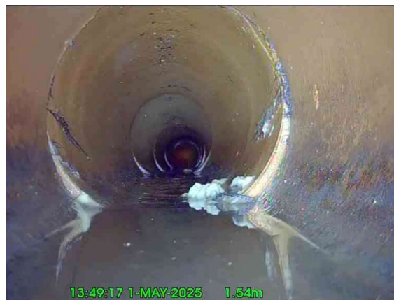
2, 00:00:17, 1.54 m Roots, fine at joint
