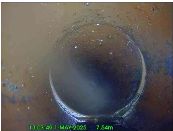
3, 00:00:42, 7.54 m Joint displaced, medium
