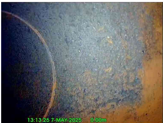
1, 00:00:06, 0.00 m Line deviates left
