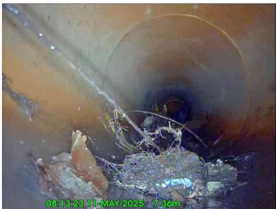
3, 00:01:49, 7.36 m Settled deposits, coarse, 5% cross-sectional area loss
