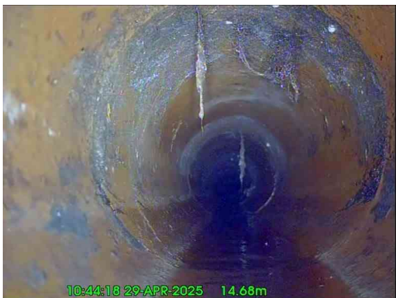
13, 00:01:36, 14.68 m Roots, fine at joint
