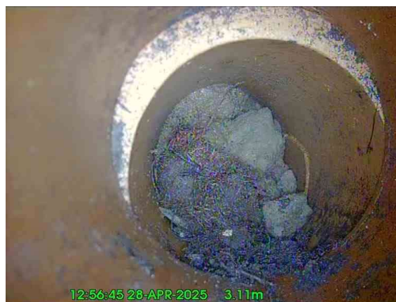
4, 00:00:30, 3.11 m Joint displaced, medium
