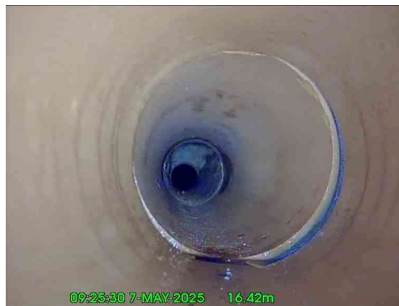
8, 00:01:06, 16.42 m Joint displaced, medium
