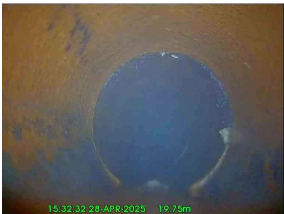
5, 00:01:33, 19.75 m Roots, mass at joint, 5% cross-sectional area loss, start
