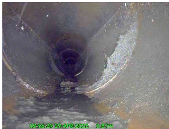
2, 00:00:10, 0.87 m Roots, mass at joint, 5% cross-sectional area loss
