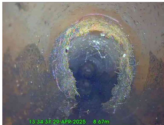
4, 00:00:52, 8.67 m Roots, mass at joint, 20% cross-sectional area loss
