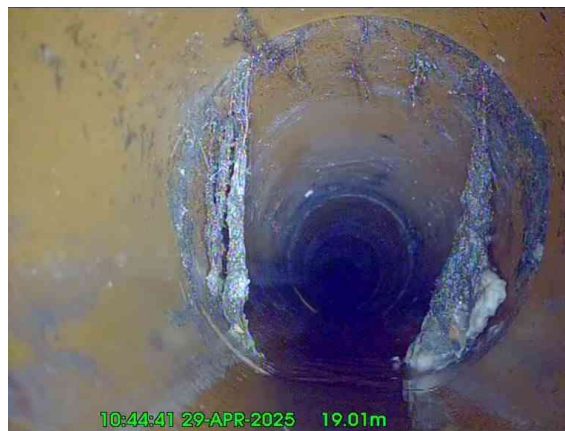
16, 00:01:59, 19.01 m Roots, mass at joint, 10% cross-sectional area loss
