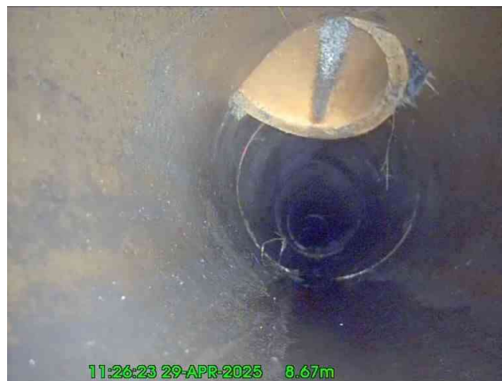
6, 00:00:41, 8.67 m Roots, fine, Intruding via connection
