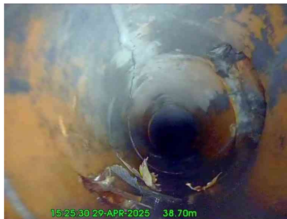
8, 00:03:03, 38.70 m Connection other than junction at 2 o'clock, 100mm dia
