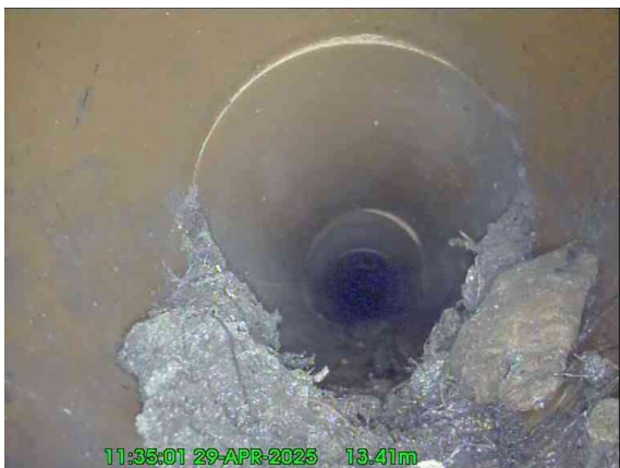
5, 00:02:02, 13.41 m Roots, mass at joint, 10% cross-sectional area loss
