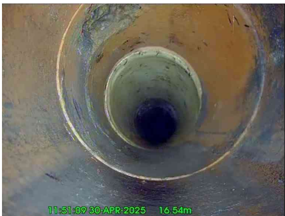
3, 00:00:47, 16.54 m Surface damage, increased roughness from 10 o'clock to 11 o'clock
