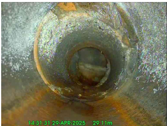
5, 00:01:47, 29.11 m Surface damage, increased roughness from 10 o'clock to 3 o'clock
