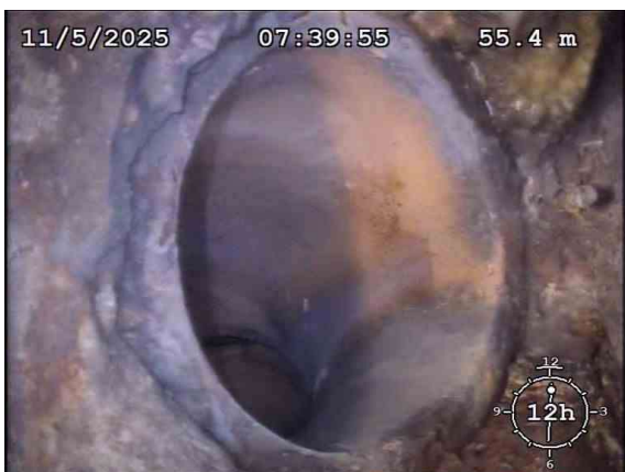
13, 00:06:12, 55.40 m Connection other than junction at 11 o'clock, 150mm dia
