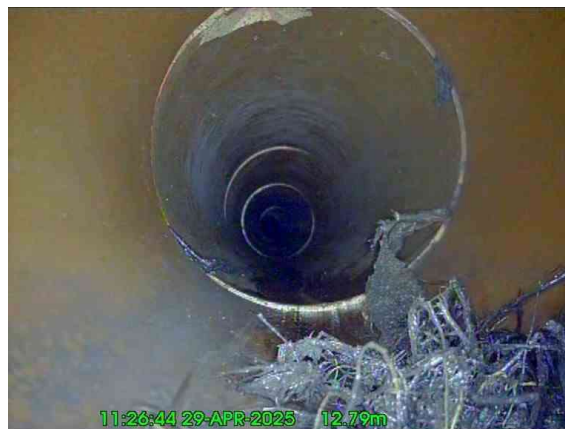
10, 00:01:01, 12.79 m Roots, mass at joint, 5% cross-sectional area loss
