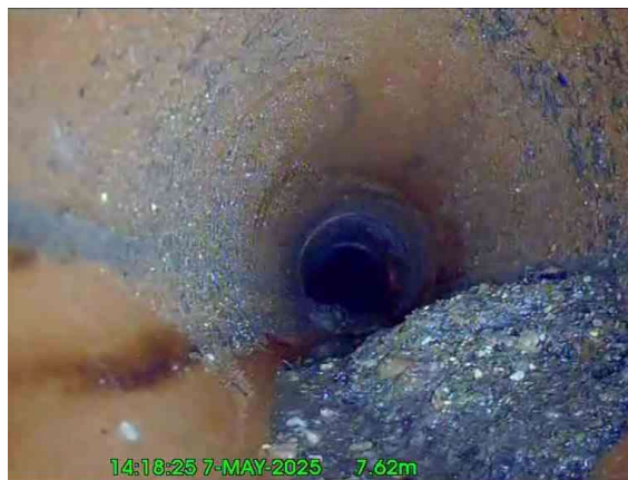
4, 00:00:38, 7.62 m Settled deposits, fine, 10% cross-sectional area loss, start
