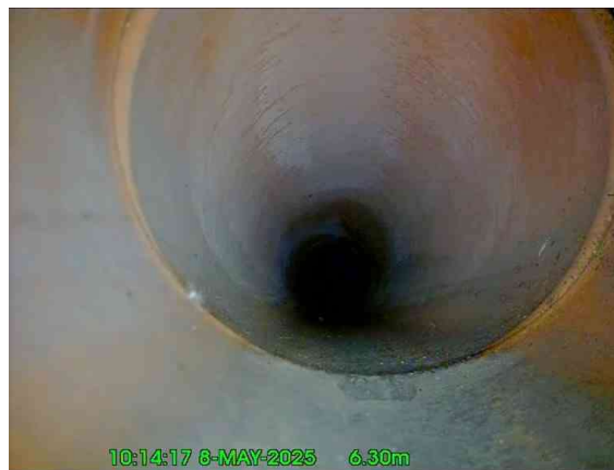
4, 00:00:25, 6.30 m Line deviates down
