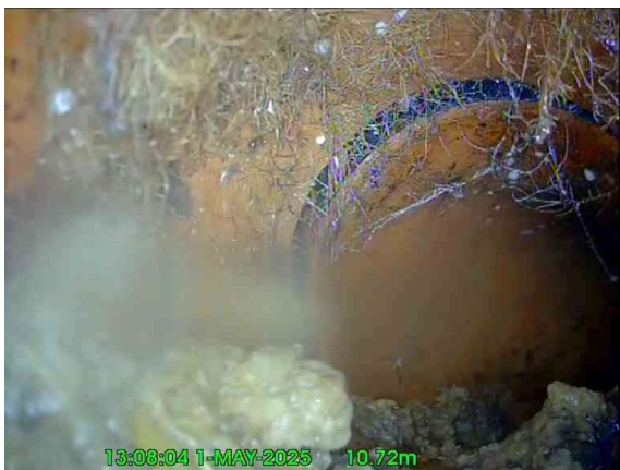
7, 00:00:57, 10.72 m Joint displaced, medium
