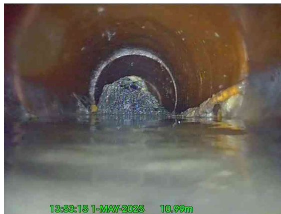
10, 00:02:12, 10.99 m Roots, tap at joint
