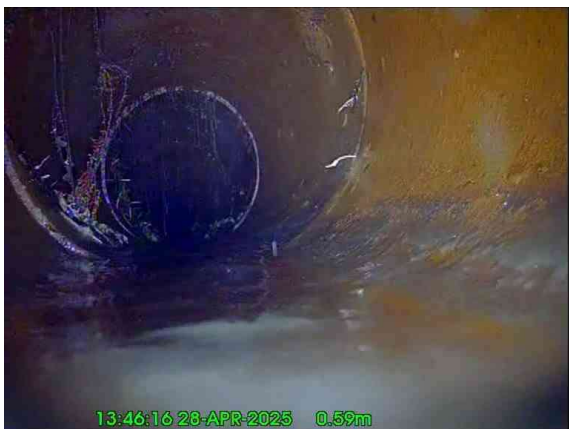
1, 00:00:07, 0.59 m Roots, mass at joint, 5% cross-sectional area loss, start
