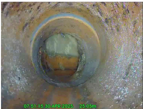
7, 00:01:17, 25.05 m Joint displaced, medium
