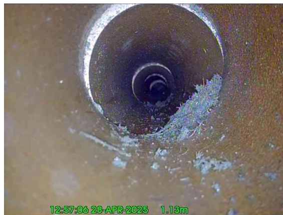
2, 00:00:51, 1.13 m Roots, mass at joint, 5% cross-sectional area loss
