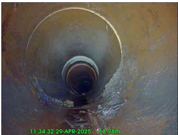
7, 00:01:33, 18.98 m Roots, mass at joint, 5% cross-sectional area loss
