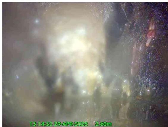
2, 00:01:58, 3.60 m Roots, mass at joint, 75% cross-sectional area loss
