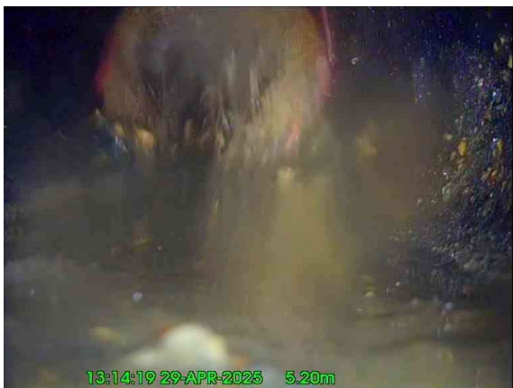
3, 00:01:44, 5.20 m Roots, mass at joint, 35% cross-sectional area loss
