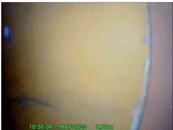
1, 00:00:02, 0.00 m Line deviates left
