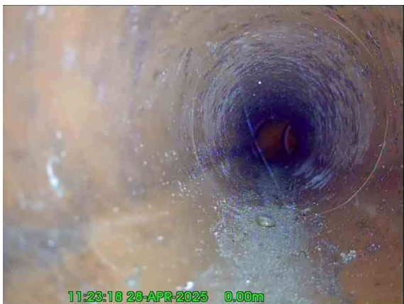
1, 00:00:01, 0.00 m Crack, circumferential from 1 o'clock to 5 o'clock
