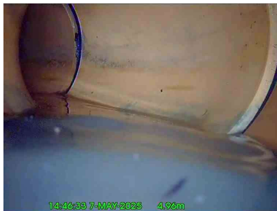
2, 00:00:26, 4.96 m Line deviates left
