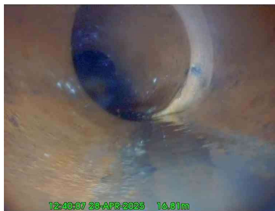
4, 00:01:17, 16.81 m Line deviates left
