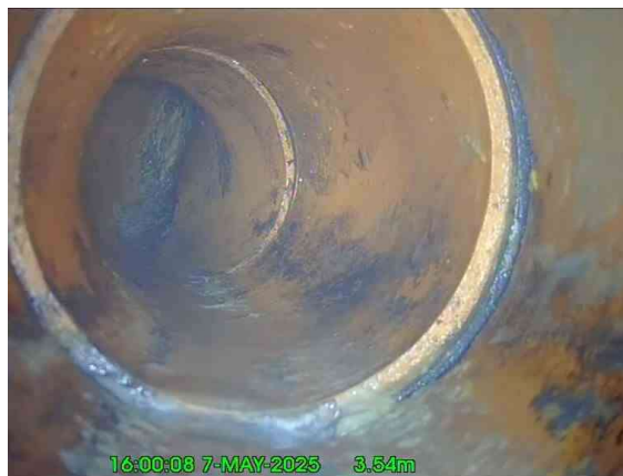
2, 00:00:28, 3.54 m Joint displaced, medium
