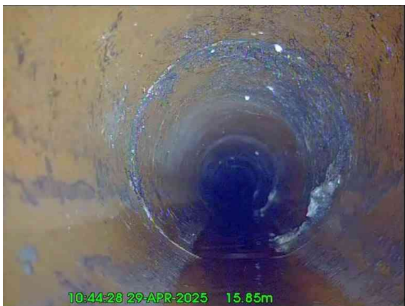
15, 00:01:46, 15.85 m Roots, mass at joint, 5% cross-sectional area loss
