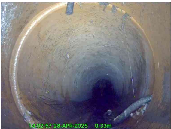
1, 00:00:06, 0.33 m Roots, tap at joint
