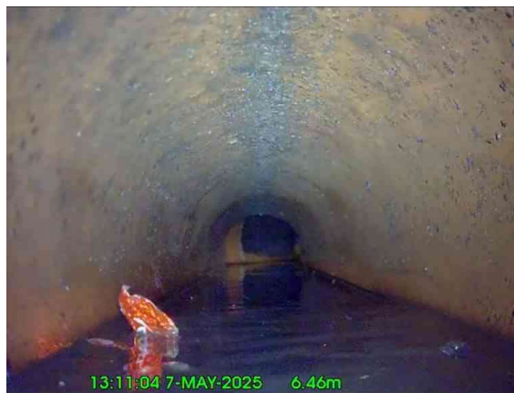
4, 00:00:19, 6.46 m Water level, 20% of the vertical dimension, Water standing in sewer
