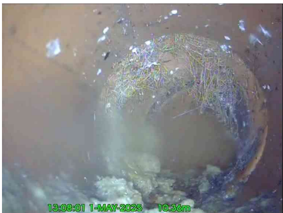
5, 00:00:54, 10.36 m Roots, mass at joint, 10% cross-sectional area loss
