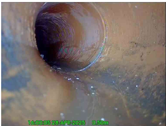
3, 00:00:13, 0.50 m Line deviates left
