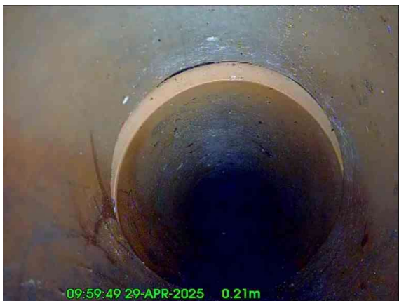
1, 00:00:06, 0.21 m Joint displaced, medium
