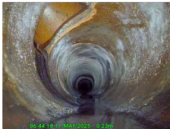
2, 00:00:06, 0.23 m Connection other than junction at 10 o'clock, 100mm dia
