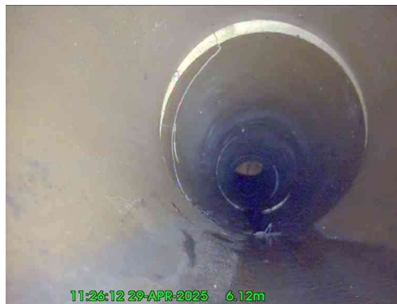
4, 00:00:30, 6.12 m Crack, circumferential at joint from 8 o'clock to 11 o'clock
