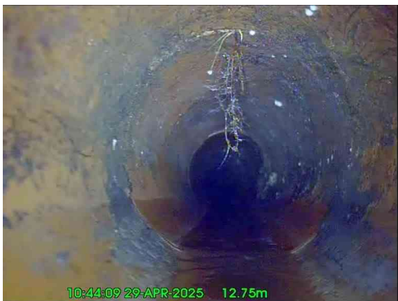
11, 00:01:27, 12.75 m Roots, fine at joint
