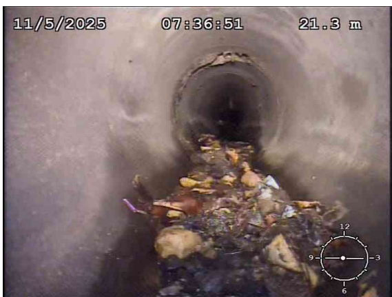
5, 00:03:08, 21.30 m Settled deposits, coarse, 10% cross-sectional area loss, start
