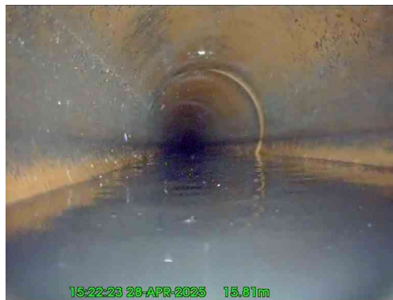
4, 00:04:14, 15.81 m Water level, 20% of the vertical dimension, Water standing in sewer
