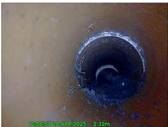
3, 00:00:38, 2.32 m Roots, mass at joint, 10% cross-sectional area loss
