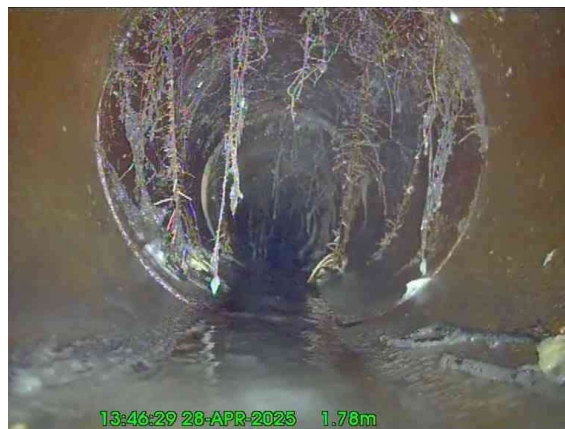
2, 00:00:20, 1.78 m Roots, mass at joint, 10% cross-sectional area loss, change
