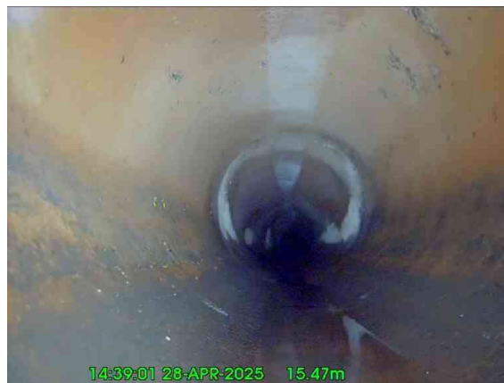
6, 00:01:27, 15.47 m Settled deposits, coarse, 5% cross-sectional area loss, finish
