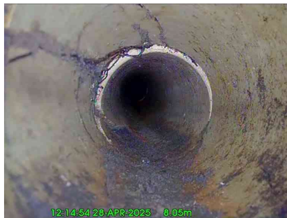
10, 00:01:09, 8.05 m Roots, fine at joint
