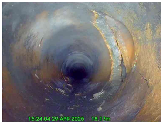
4, 00:01:38, 18.17 m Connection other than junction at 2 o'clock, 100mm dia
