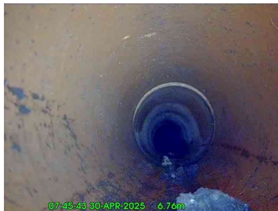
2, 00:00:27, 6.76 m Settled deposits, fine, 5% cross-sectional area loss, change
