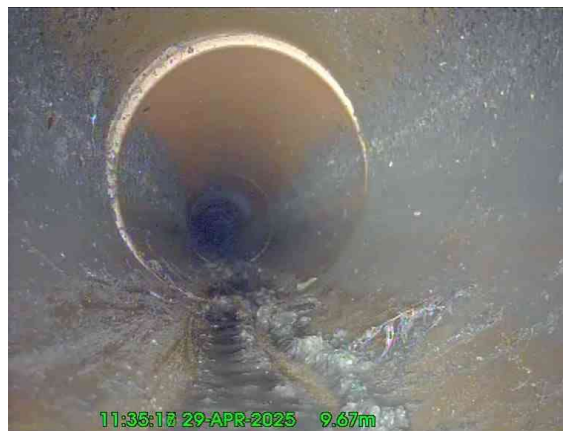
4, 00:02:19, 9.67 m Roots, mass at joint, 20% cross-sectional area loss, finish
