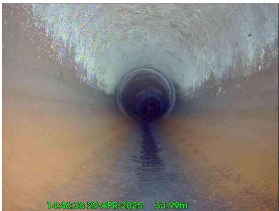
7, 00:01:22, 33.99 m Survey abandoned, Unable to push camera any further
