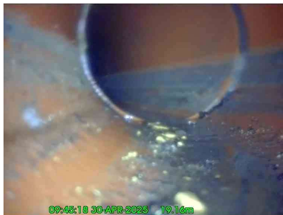
10, 00:00:20, 19.16 m Line deviates left
