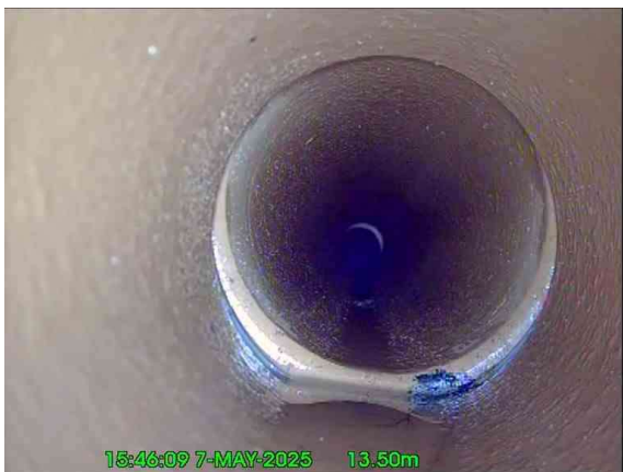
3, 00:01:00, 13.50 m Joint displaced, medium
