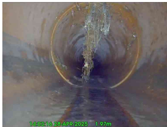
2, 00:00:25, 1.97 m Roots, mass at joint, 5% cross-sectional area loss
