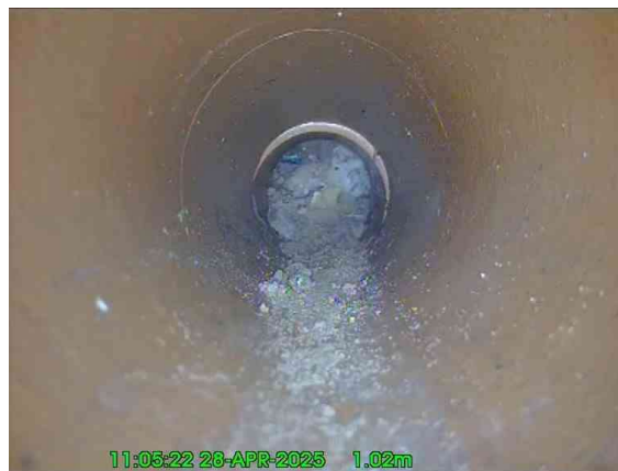
2, 00:00:14, 1.02 m Crack, circumferential from 8 o'clock to 3 o'clock
