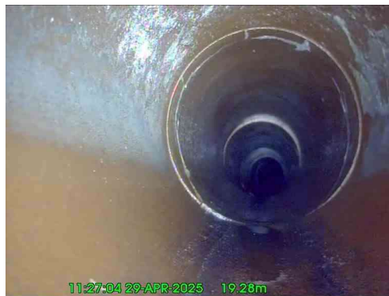
12, 00:01:21, 19.28 m Crack, circumferential at joint from 8 o'clock to 4 o'clock
