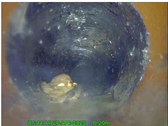
07:44:19 29-APR-2025 0.20m 1, 00:00:06, 0.20 m Pipe material changes to pitch fibre at this point
