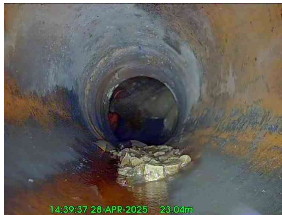
8, 00:02:03, 23.04 m Settled deposits, coarse, 5% cross-sectional area loss
