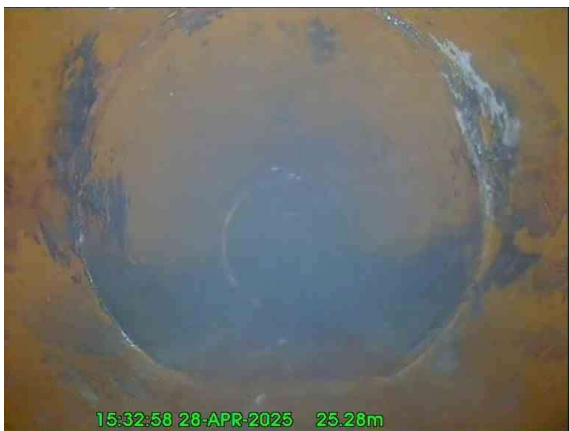
7, 00:01:59, 25.28 m Roots, mass at joint, 5% cross-sectional area loss, finish
