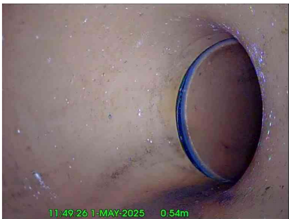
3, 00:00:11, 0.54 m Joint displaced, medium
