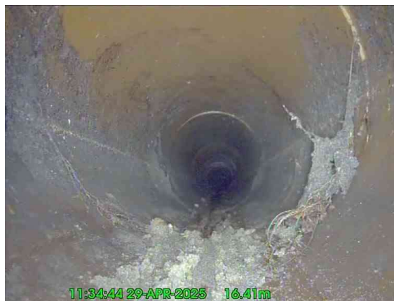
6, 00:01:45, 16.41 m Roots, fine at joint
