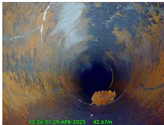
10, 00:03:34, 42.67 m Survey abandoned, Unable to push camera any further
