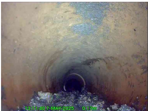
1, 00:00:55, 0.17 m Settled deposits, coarse, 10% cross-sectional area loss, start
