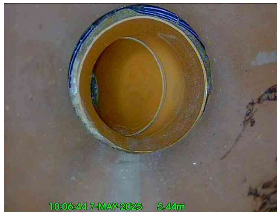
4, 00:00:36, 5.44 m Joint displaced, medium
