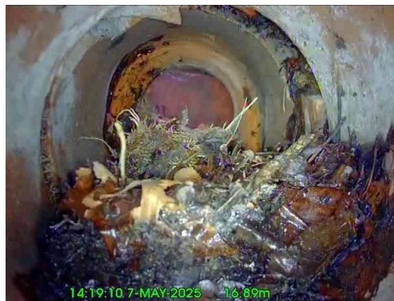
8, 00:01:25, 16.89 m Roots, mass at joint, 25% cross-sectional area loss, At entry to gully
