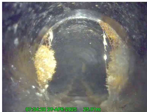
6, 00:01:55, 25.91 m Roots, mass at joint, 10% cross-sectional area loss
