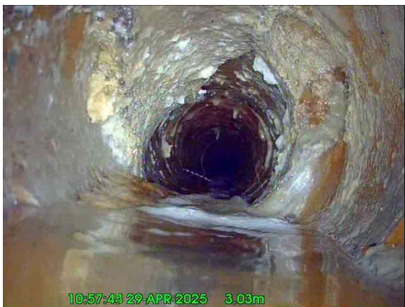
3, 00:00:26, 3.03 m Attached deposits, grease from 8 o'clock to 4 o'clock, 10% cross-sectional area loss
