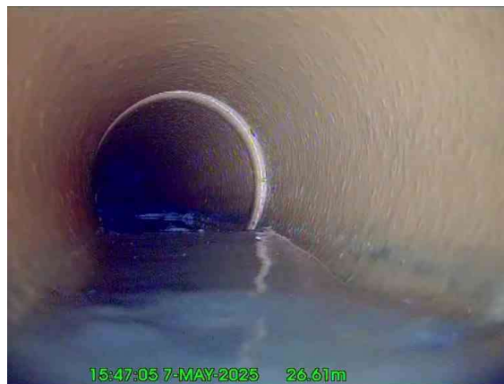
6, 00:01:55, 26.61 m Line deviates left
