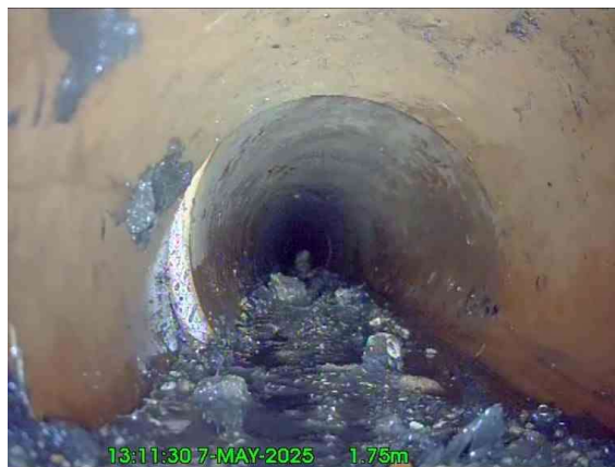
2, 00:00:45, 1.75 m Joint displaced, medium
