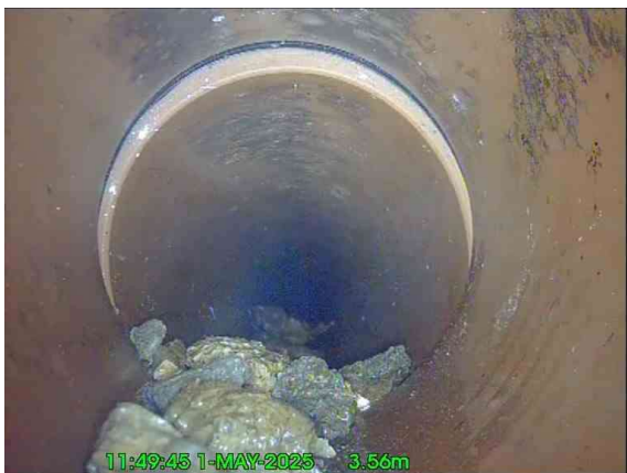
5, 00:00:30, 3.56 m Joint displaced, medium
