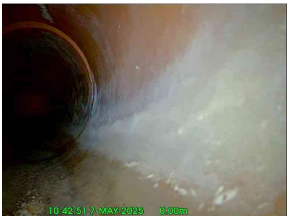
1, 00:00:02, 0.00 m Line deviates left
