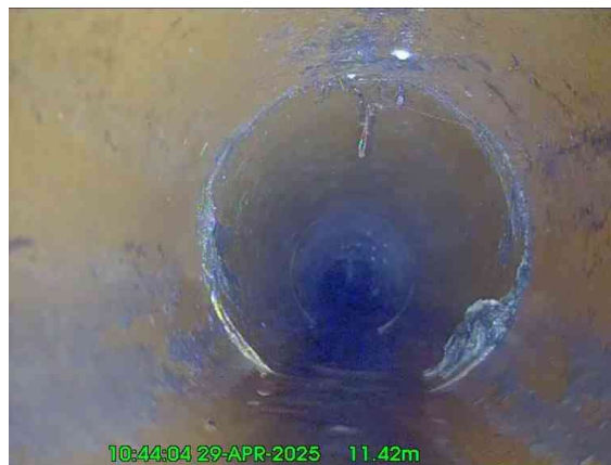
10, 00:01:22, 11.42 m Roots, mass at joint, 5% cross-sectional area loss
