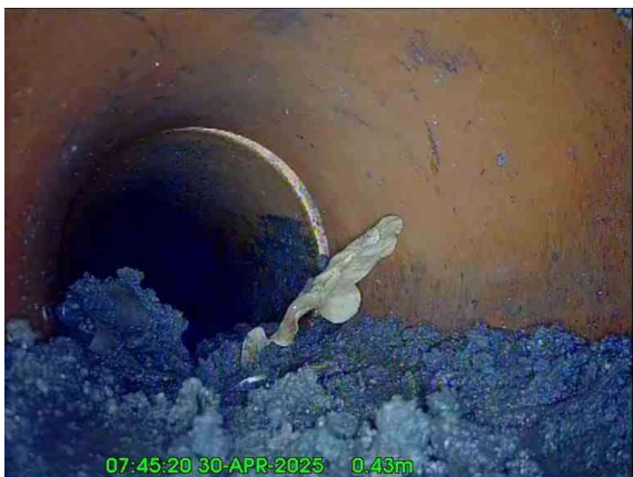
1, 00:00:04, 0.43 m Settled deposits, fine, 10% cross-sectional area loss, start
