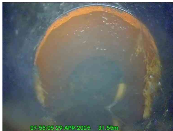
10, 00:02:40, 31.55 m Roots, mass at joint, 5% cross-sectional area loss
