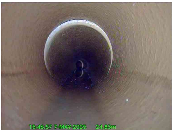
5, 00:01:46, 24.83 m Joint displaced, medium
