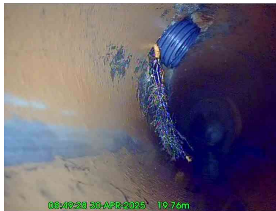
4, 00:01:24, 19.76 m Roots, mass, 5% cross-sectional area loss, Intruding via connection
