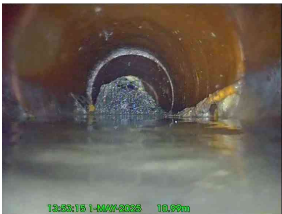
11, 00:02:12, 10.99 m Roots, mass at joint, 35% cross-sectional area loss
