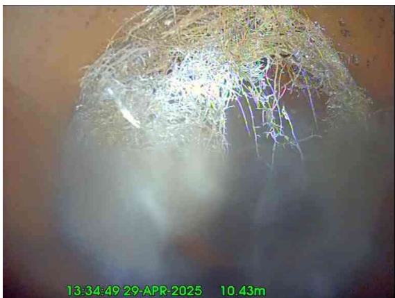
5, 00:01:04, 10.43 m Roots, mass at joint, 35% cross-sectional area loss
